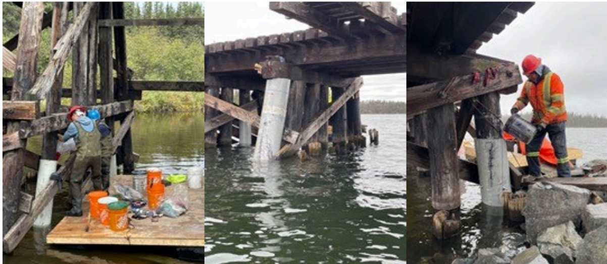
Photo: Installing the laminates to create a partial or full height repair of a pile and pouring low viscosity resin in the annular space.
