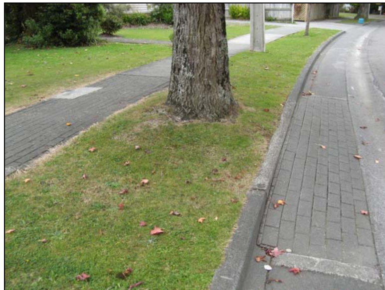
Local kerb and footpath renovation using material which accommodates some further expansion of root structure
