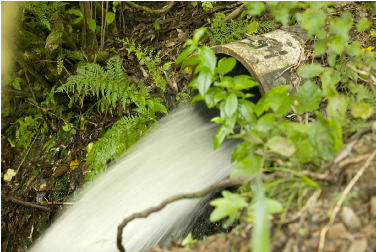
Stormwater outlet in native bush
