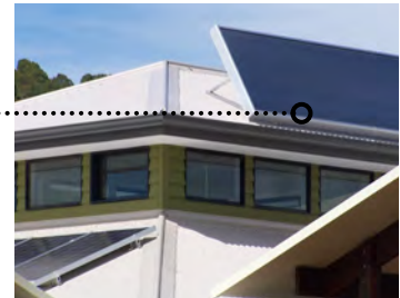
Solar collector devices positioned to maximise sunlight absorption
