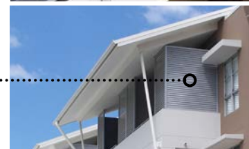
Eaves and moveable vertical shading device (external venetian blind) on east or west facing windows
