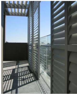
Adjustable screens enable privacy and management of sunlight access/solar gain to residential development (apartment)
