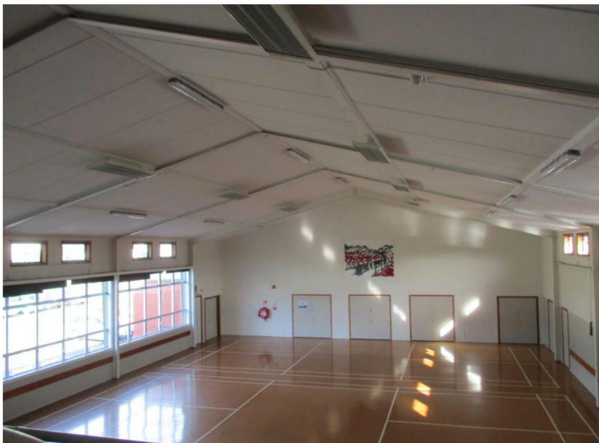
Figure 3 View of the steel portal frames in the main hall with infill timber walls
