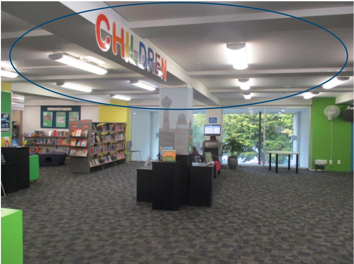
Example of reinforced concrete floor slabs on series of primary and secondary beams
