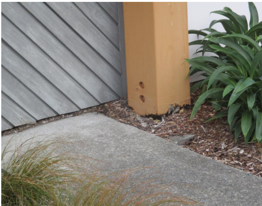
Figure 5 Degradation to column base
