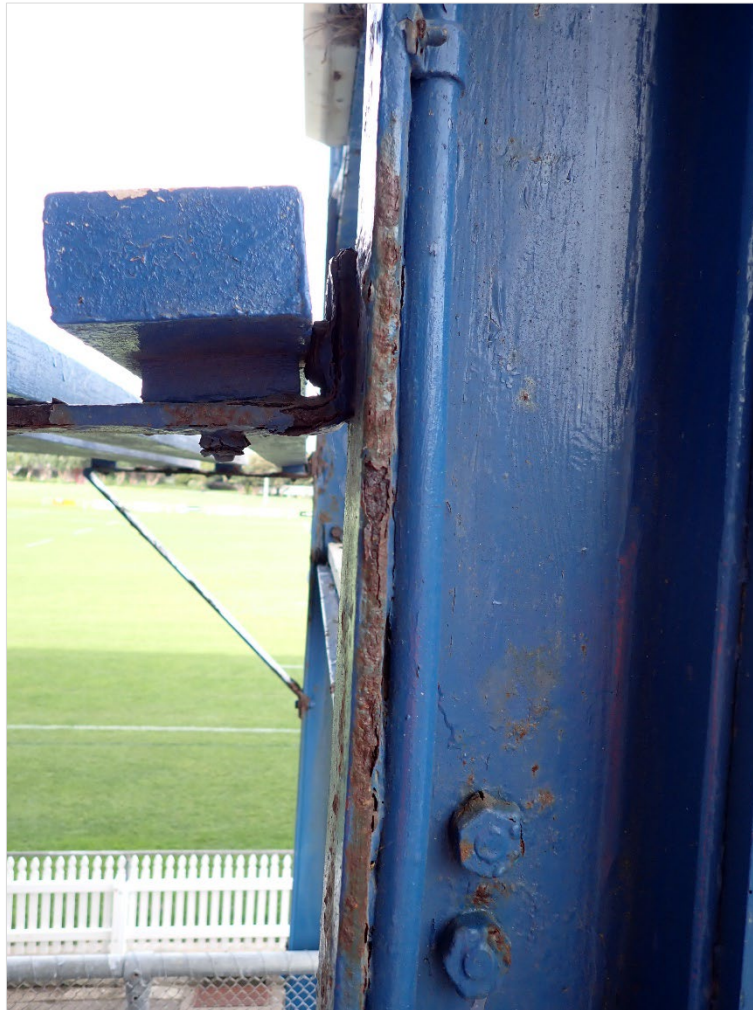
Figure 32: Item 2b – example 3, sever corrosion
