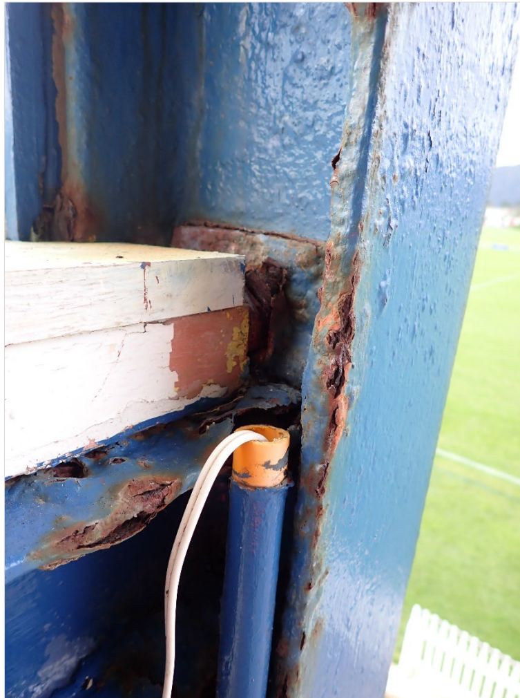
Figure 25: Item 2a – example 2, sever corrosion
