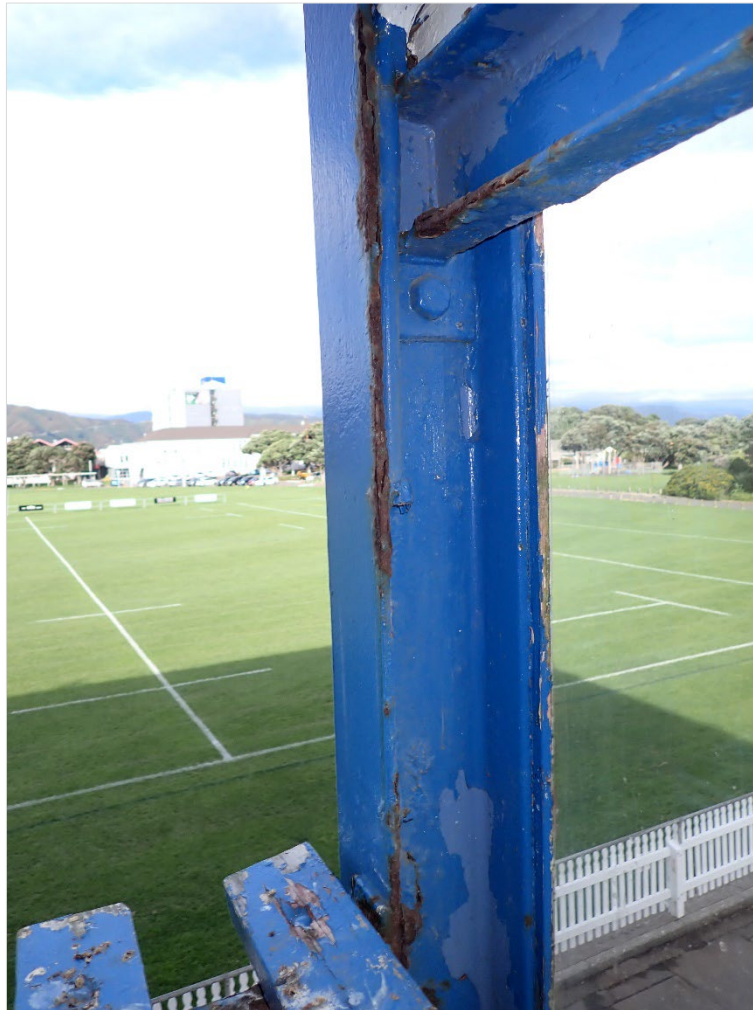
Figure 34: Item 2b – example 4, sever corrosion
