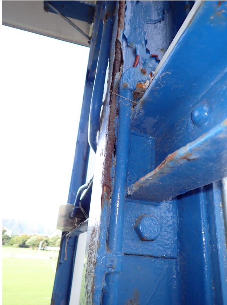
Figure 30: Item 2b – example 2, sever corrosion
