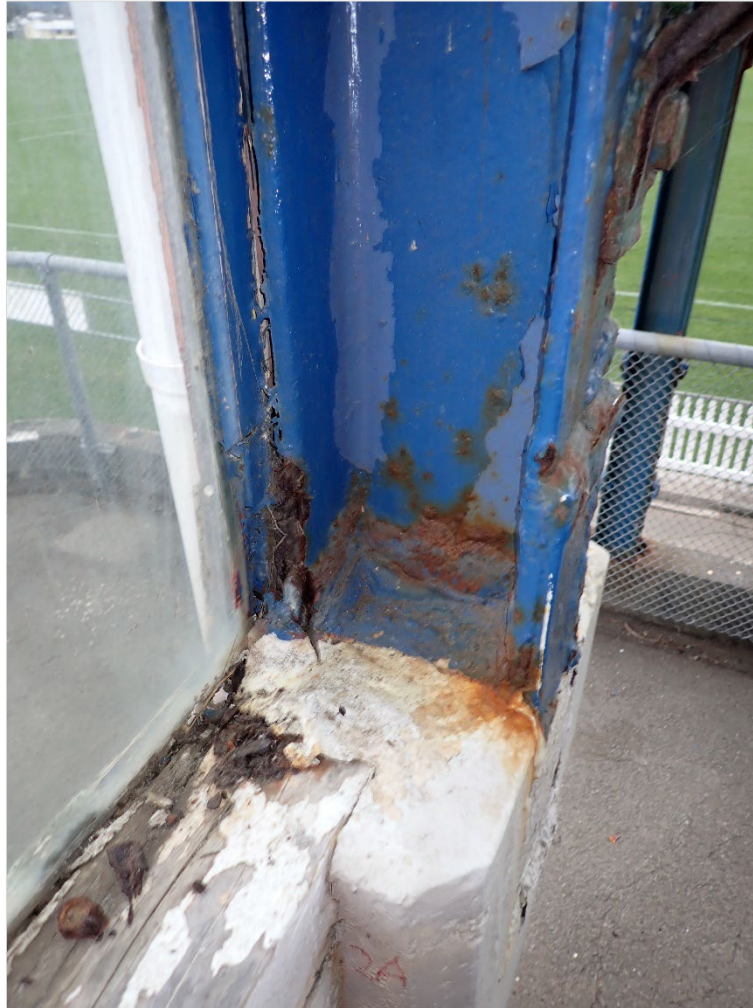
Figure 12: Location 2a - connection, sever corrosion
