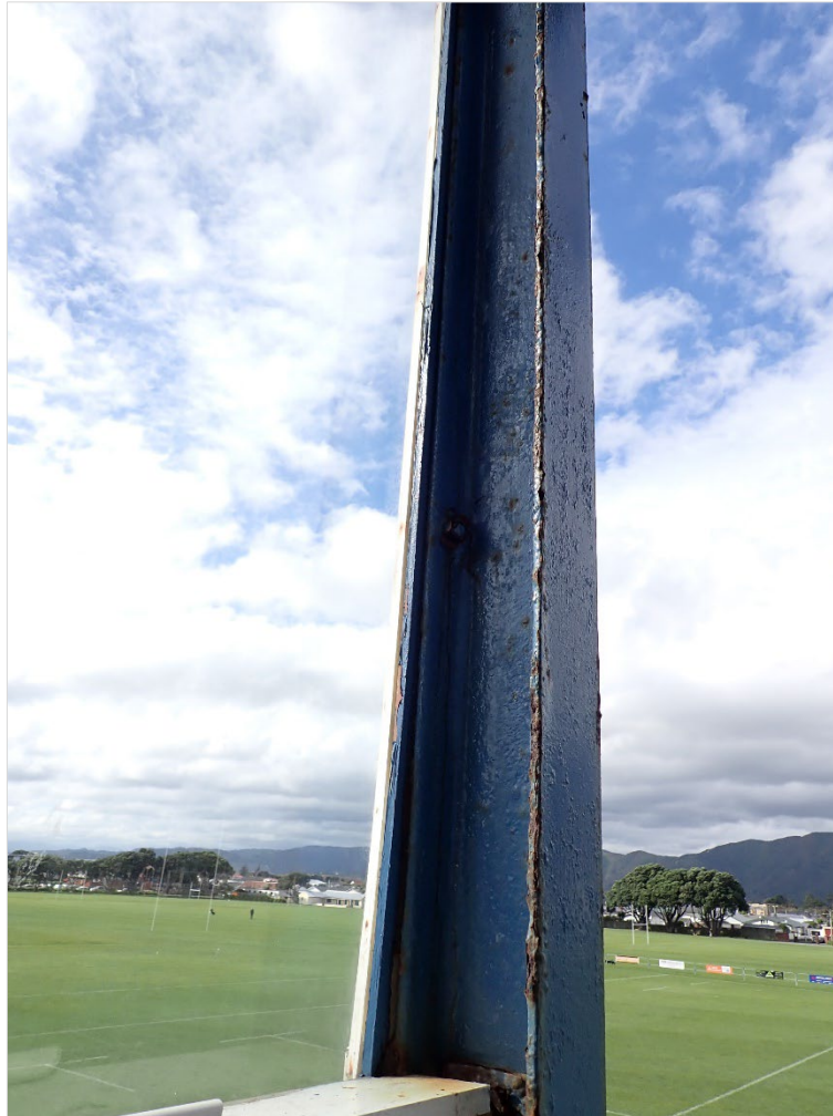
Figure 26: Item 2a – example 3, sever corrosion
