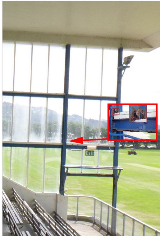
Figure 22: Item 2a – example 1, sever corrosion
