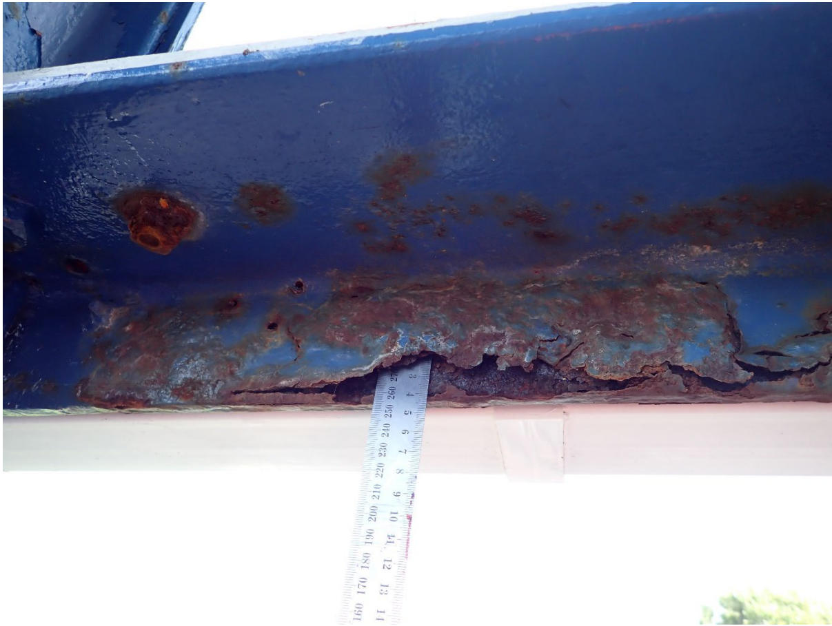
Figure 28: Item 2b – example 1, sever corrosion
