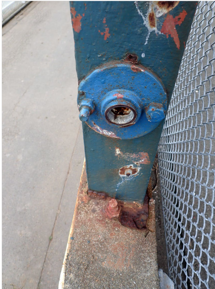
Figure 16: Grid F/X - connection, sever corrosion
