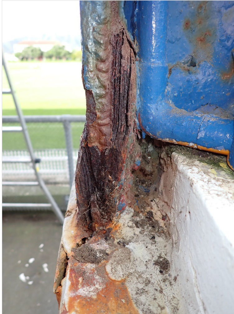
Figure 18: Location 2b - connection, sever corrosion
