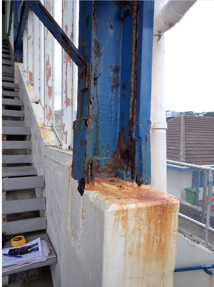
Figure 11: Location 2a - connection, sever corrosion
