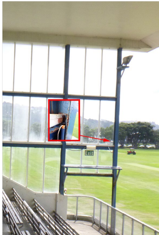
Figure 24: Item 2a – example 2, sever corrosion
