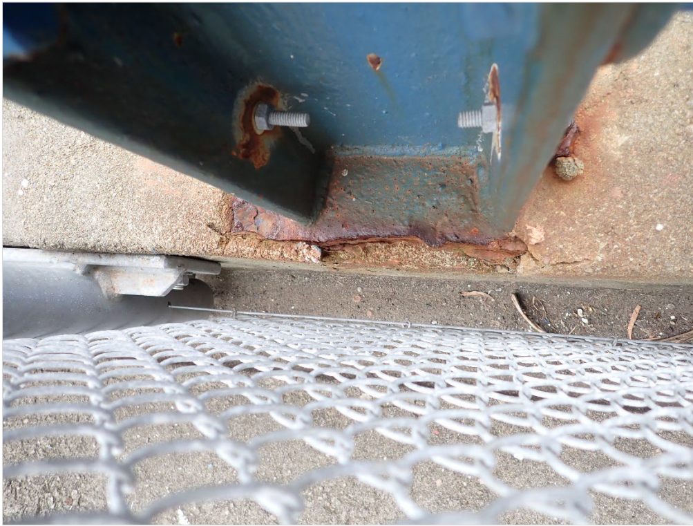
Figure 15: Grid F/X - connection, sever corrosion
