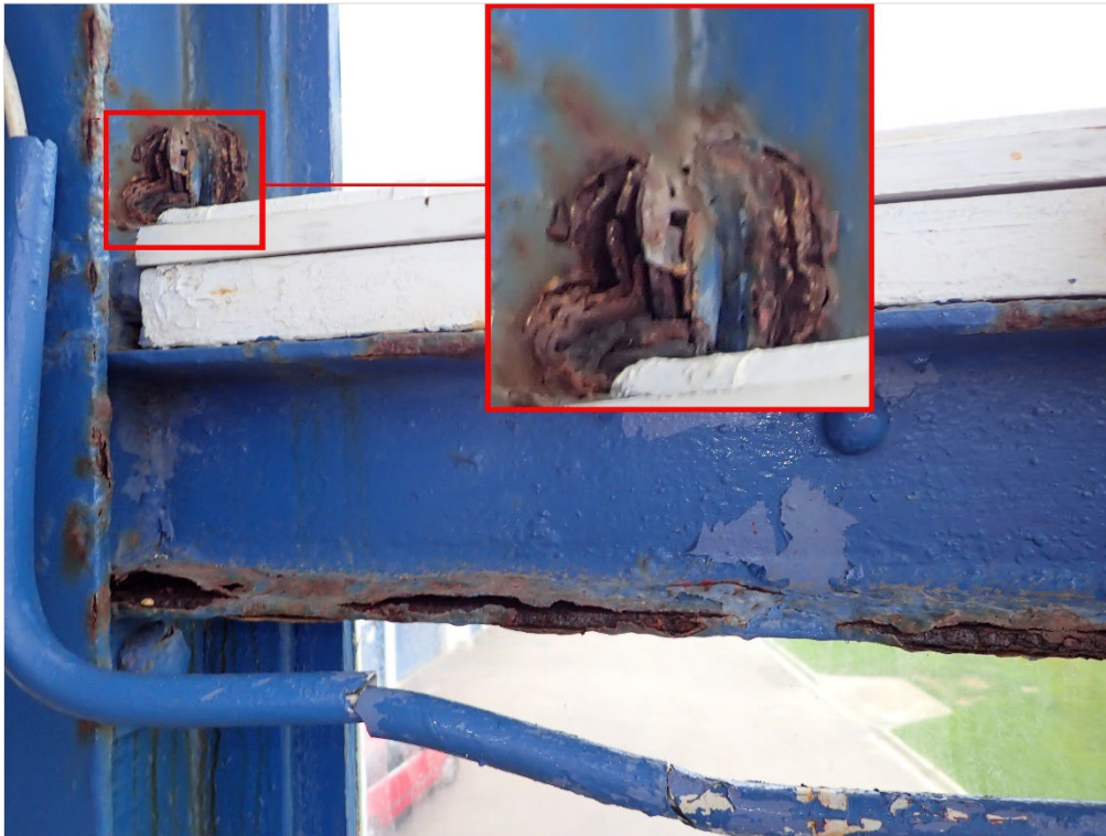
Figure 23: Item 2a – example 1, sever corrosion
