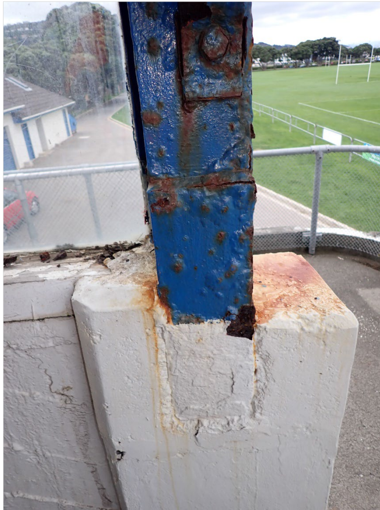
Figure 13: Location 2a - connection, sever corrosion
