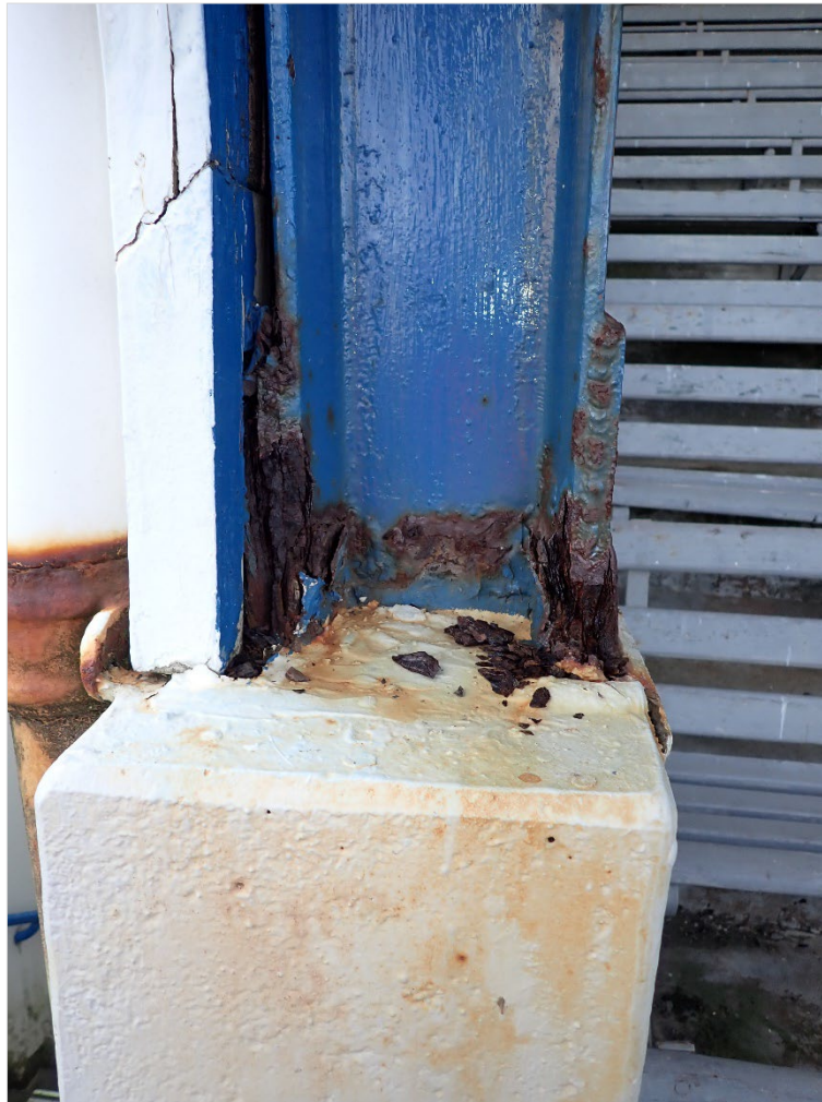
Figure 19: Location 2b - connection, sever corrosion
