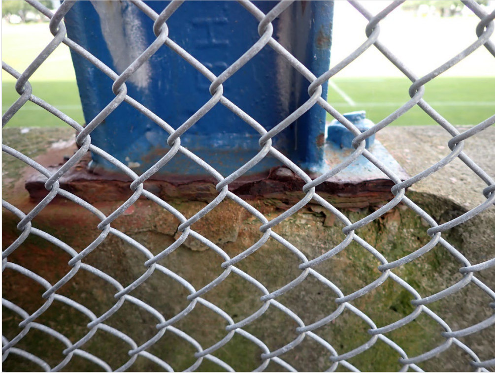
Figure 21: Grid AX - connection, sever corrosion
