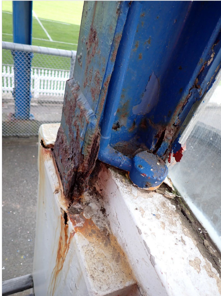
Figure 17: Location 2b - connection, sever corrosion
