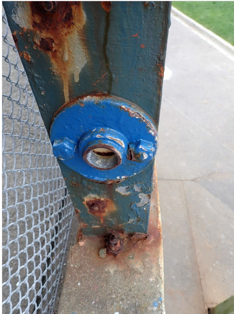
Figure 14: Grid F/X - connection, sever corrosion
