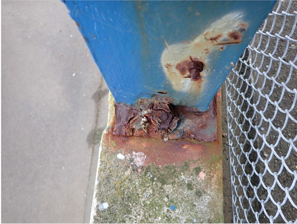
Figure 20: Grid AX - connection, sever corrosion
