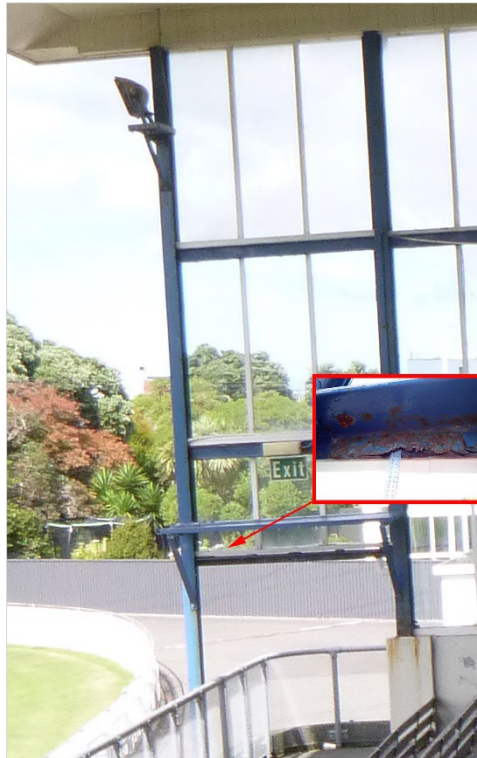
Figure 27: Item 2b – example 1, sever corrosion
