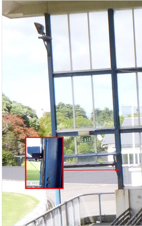
Figure 31: Item 2b – example 3, sever corrosion
