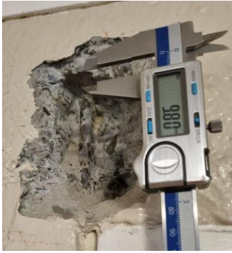
Figure 20 - Reinforcing Steel to Lintel Over the Ground Floor Corridor Adjacent to Col 10.
