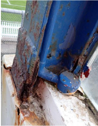
Figure 16 – Corrosion of Steel Column - Base Connection to Concrete - Column 1 Above Bleachers
