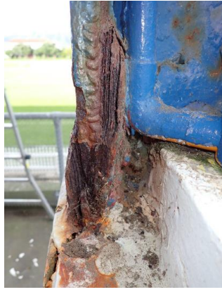
Figure 17 – Corrosion of Steel Column - Base Connection to Concrete - Column 1 Above Bleachers
