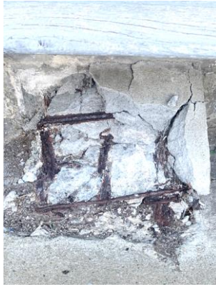
Figure 18 - Corrosion of Reinforcing Steel - Concrete Bleacher Beam - Column 3 Above Bleachers
