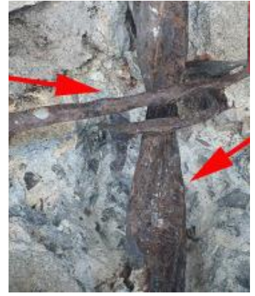
Figure 19 - Corrosion of Reinforcing Steel - Concrete Bleacher Beam - Column 3 Above Bleachers
