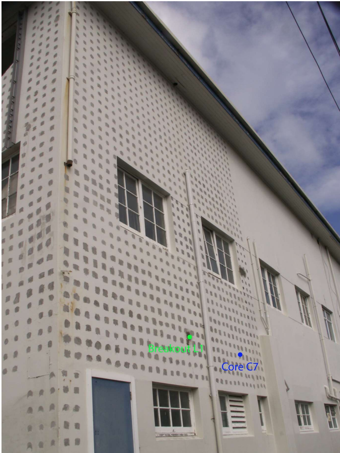
Figure 17: West Wall Grid E-F - Breakout Location
