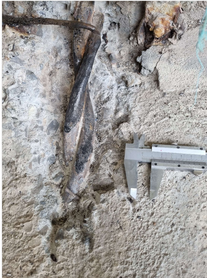
Figure 74: Raking Beam AC - Condition
