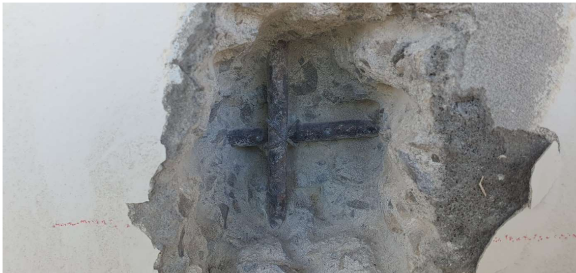
Figure 28: West Wall - Grid BC - Breakout L6
