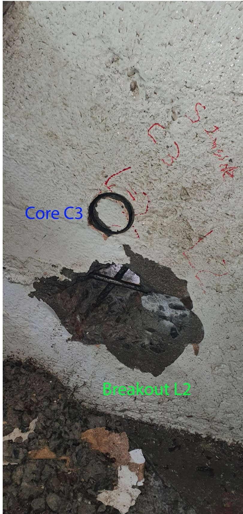
Figure 8: South Wall / North Face - Breakout L2
