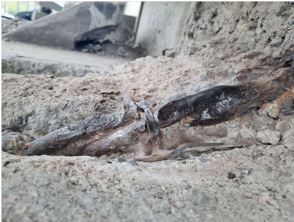
Figure 75: Raking Beam C2B - Condition
