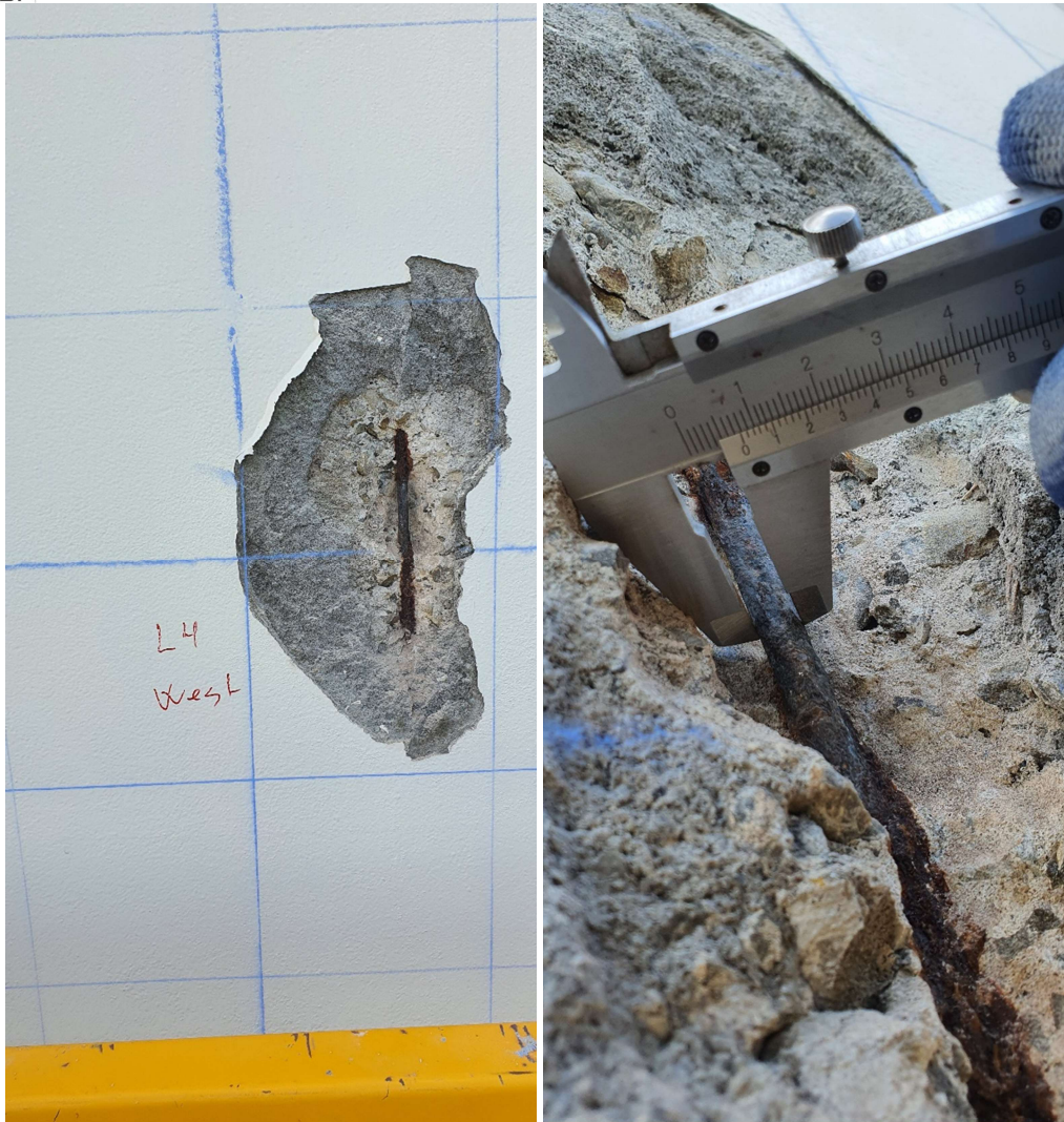
Figure 27: West Wall - Grid BC - Breakout L4
