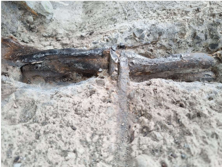
Figure 76: Raking Beam C2B - Condition
