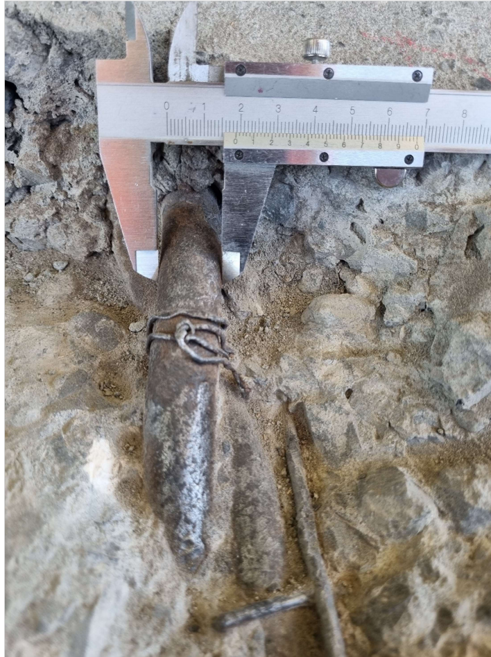
Figure 78: Raking Beam D2E - Condition
