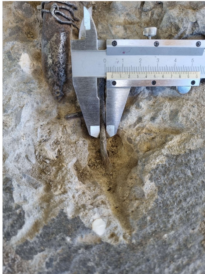
Figure 77: Raking Beam D2E - Condition
