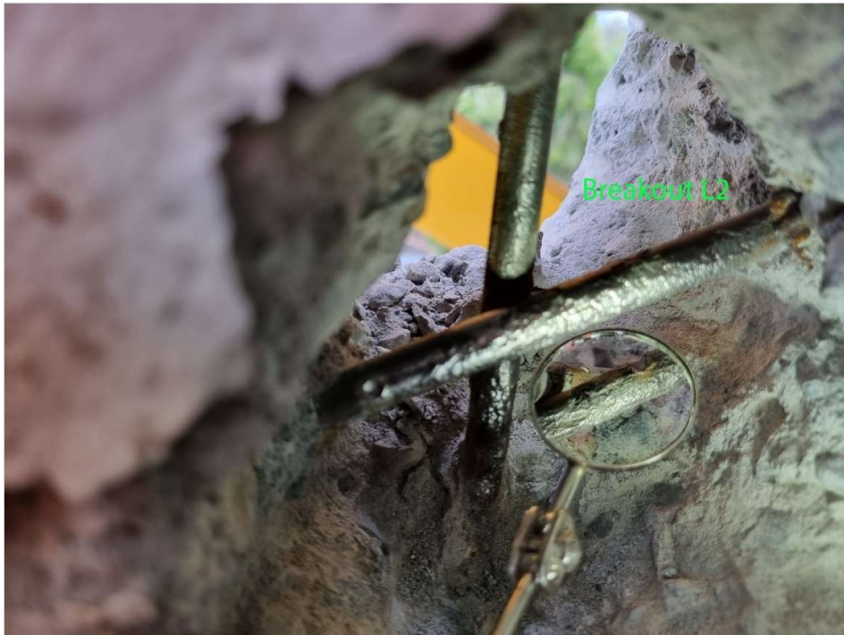
Figure 10: South Wall / North Face - Breakout L2
