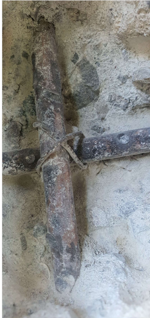
Figure 29: West Wall - Grid BC - Breakout L6
