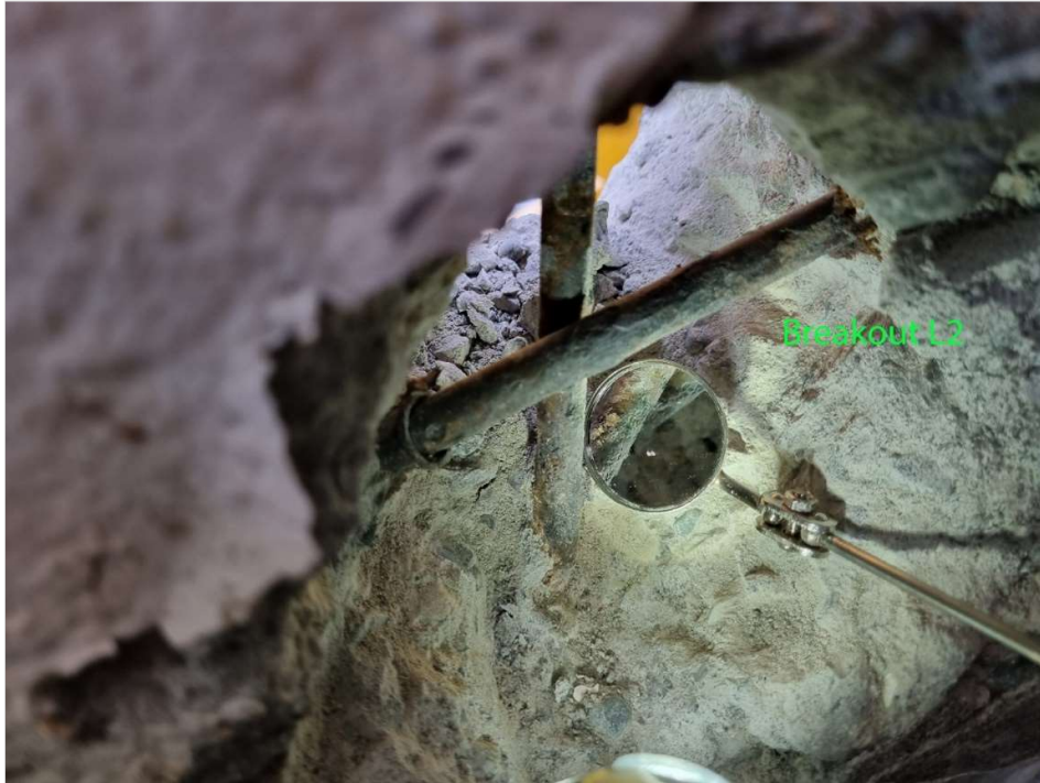
Figure 9: South Wall / North Face - Breakout L2
