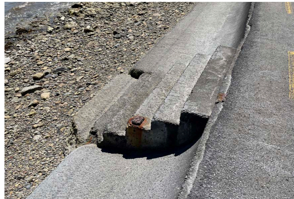
Figure 1.8 Existing steps down to beach area at Mahina Bay.
