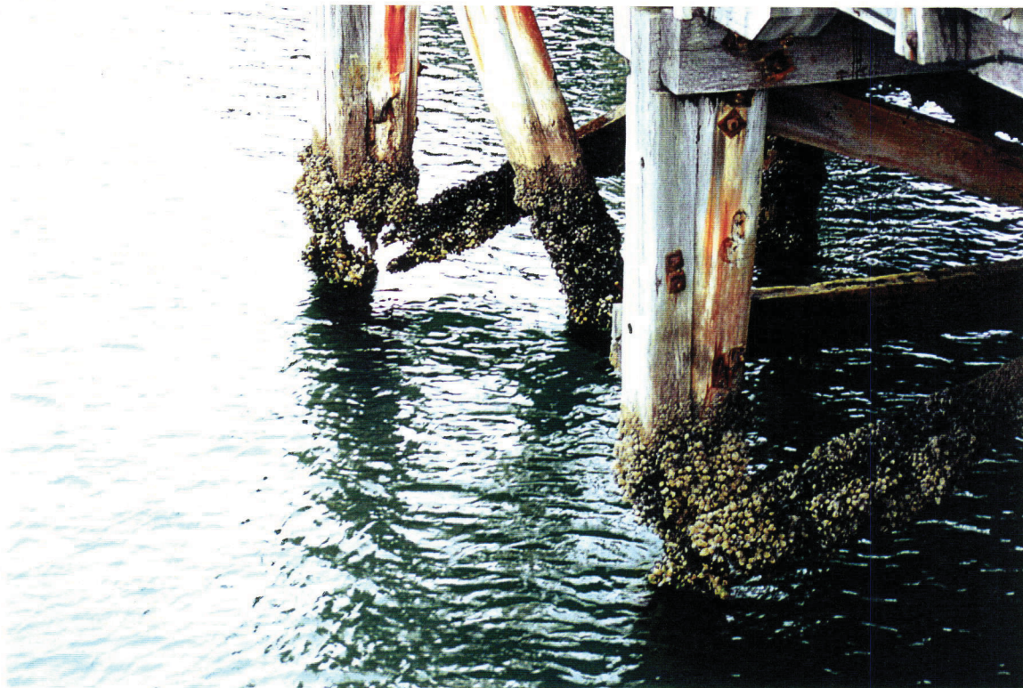
Photo 3: Corner of Central Head Pile Q38 very severely damaged
