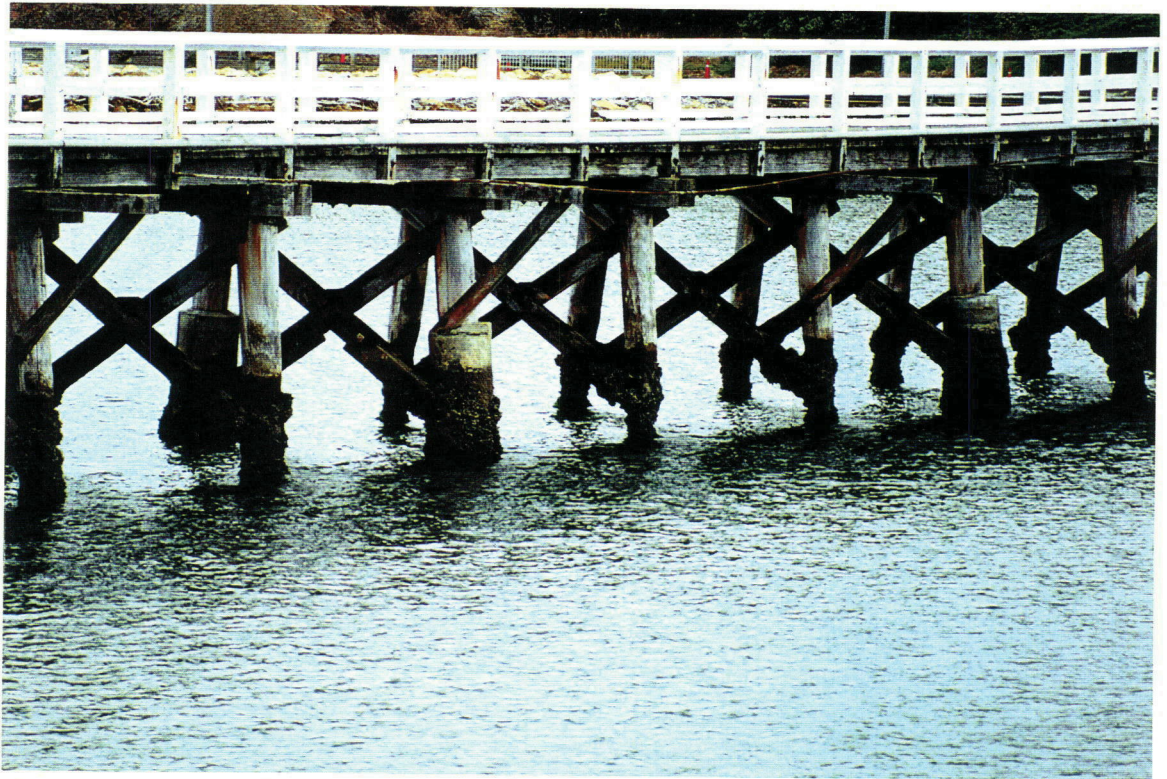
Photo 1: South side of Wharf Approach Note concrete pile jackets
