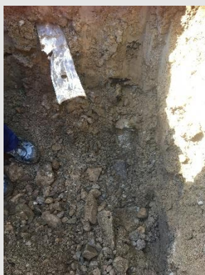
Photo 1: Location L06 - location of asbestos fibre detection (below human health criteria) (Zone 1).
