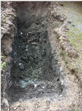
Photo 5: Location L35 – location of asbestos fibre detection (below human health criteria) (Zone 4)
