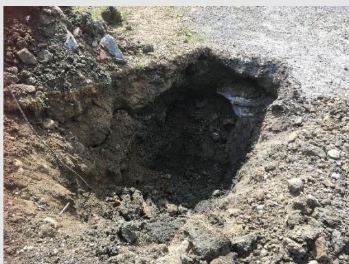
Photo 3: Location L14 – visible red brick and concrete debris (Zone 2)
