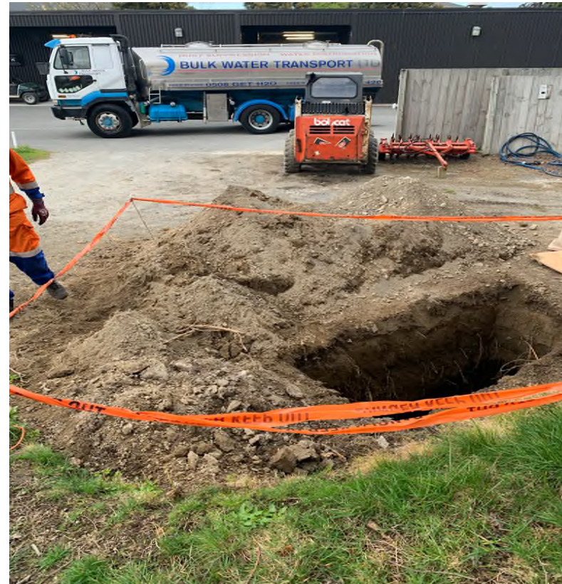
Above: View of excavated pit at test location 1 with material removed from ground shown
