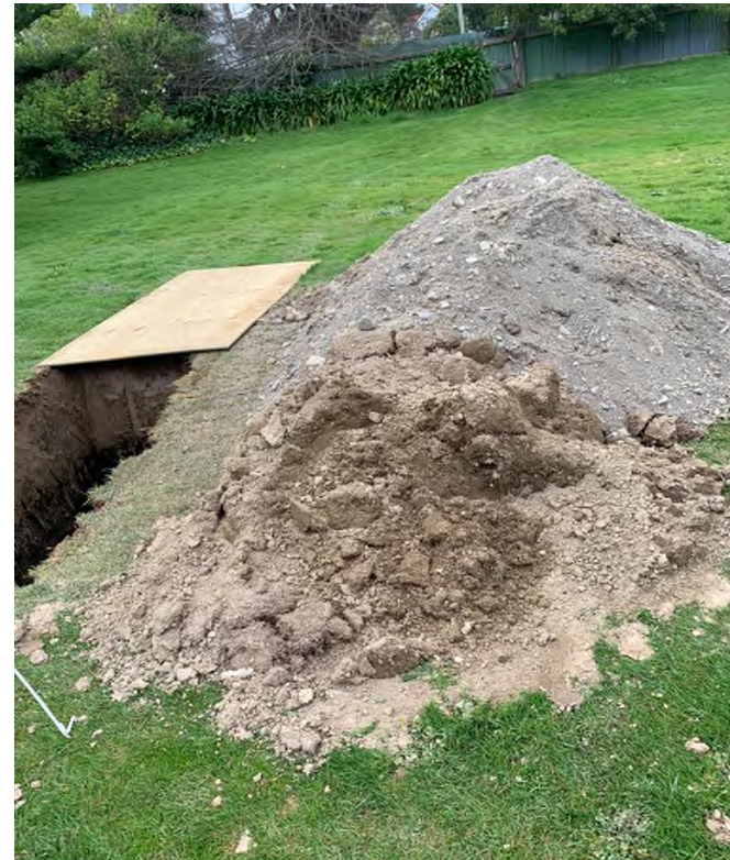
Above: View of excavated pit at test location 2 with material removed from ground shown
