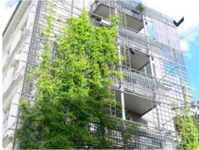
Green wall grown from base on facade framework.
