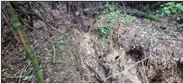
Figure 62: The upper reach of tributary 3 showing incised banks.
