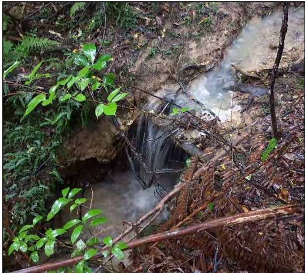
Figure 60: Ephemeral flow from stormwater discharge
