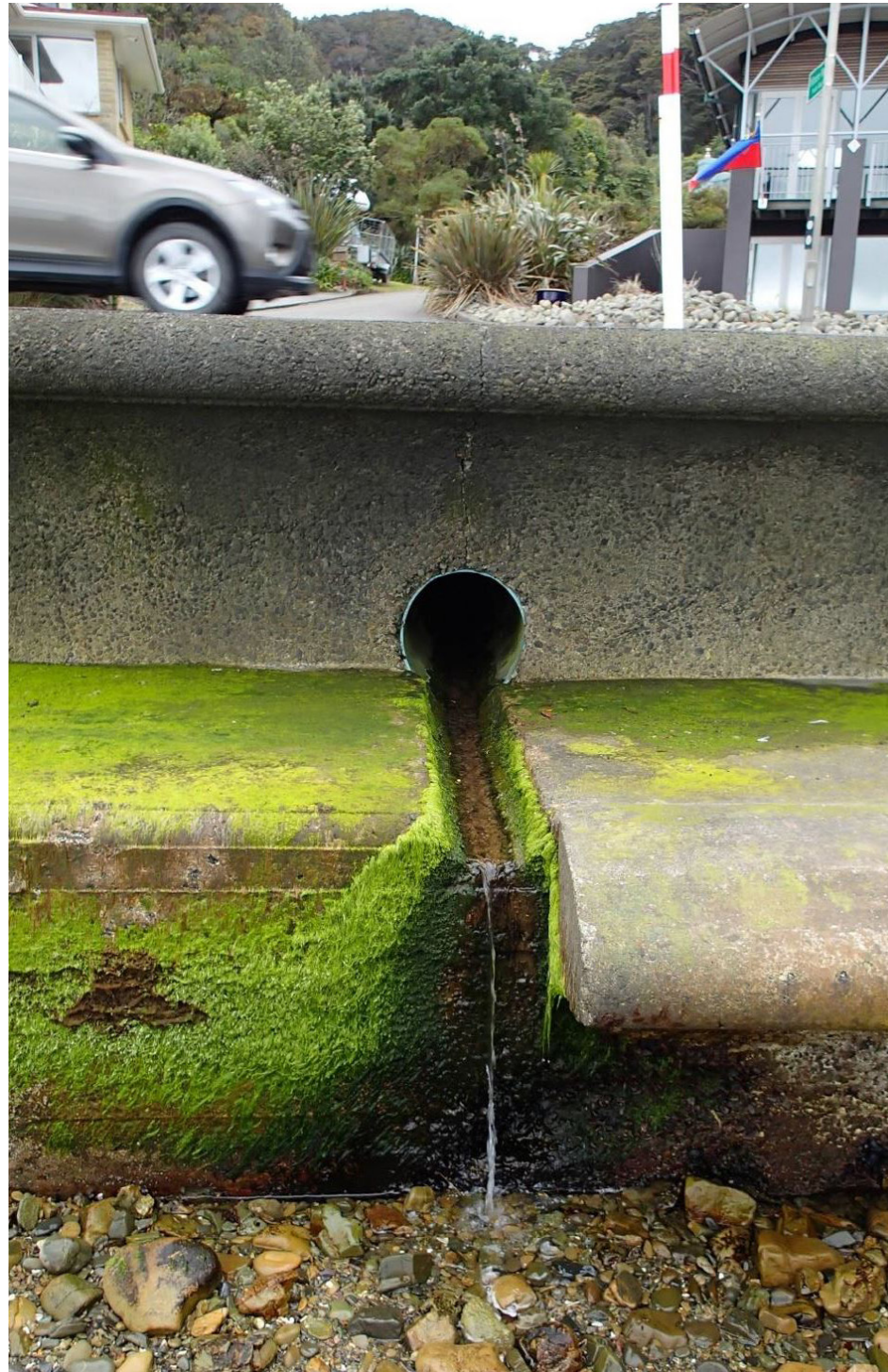
Figure 1.18 Stormwater pipe used by little penguins, Wilmore Way, northern end of Whiorau/Lowry Bay. Little penguins were reported in this drain on the inland side of the road in May 2017. Ref: Assessment of ecological effects 2019
