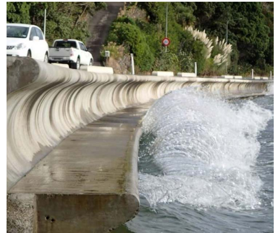
Figure 1.5 Existing double curved seawall, York Bay, built 2007–2008. Photo (taken close to high tide) Ref: Assessment of ecological effects 2019
