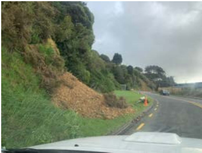
Slip at Point (4):
