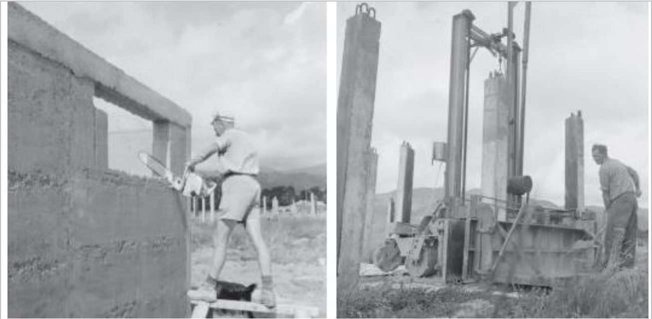
Figure 2: Constructing the Terracrete Houses, 1958. Source: Back to Earth: Earth Building in Aotearoa New Zealand 1945 – 1965 , Min Hall
