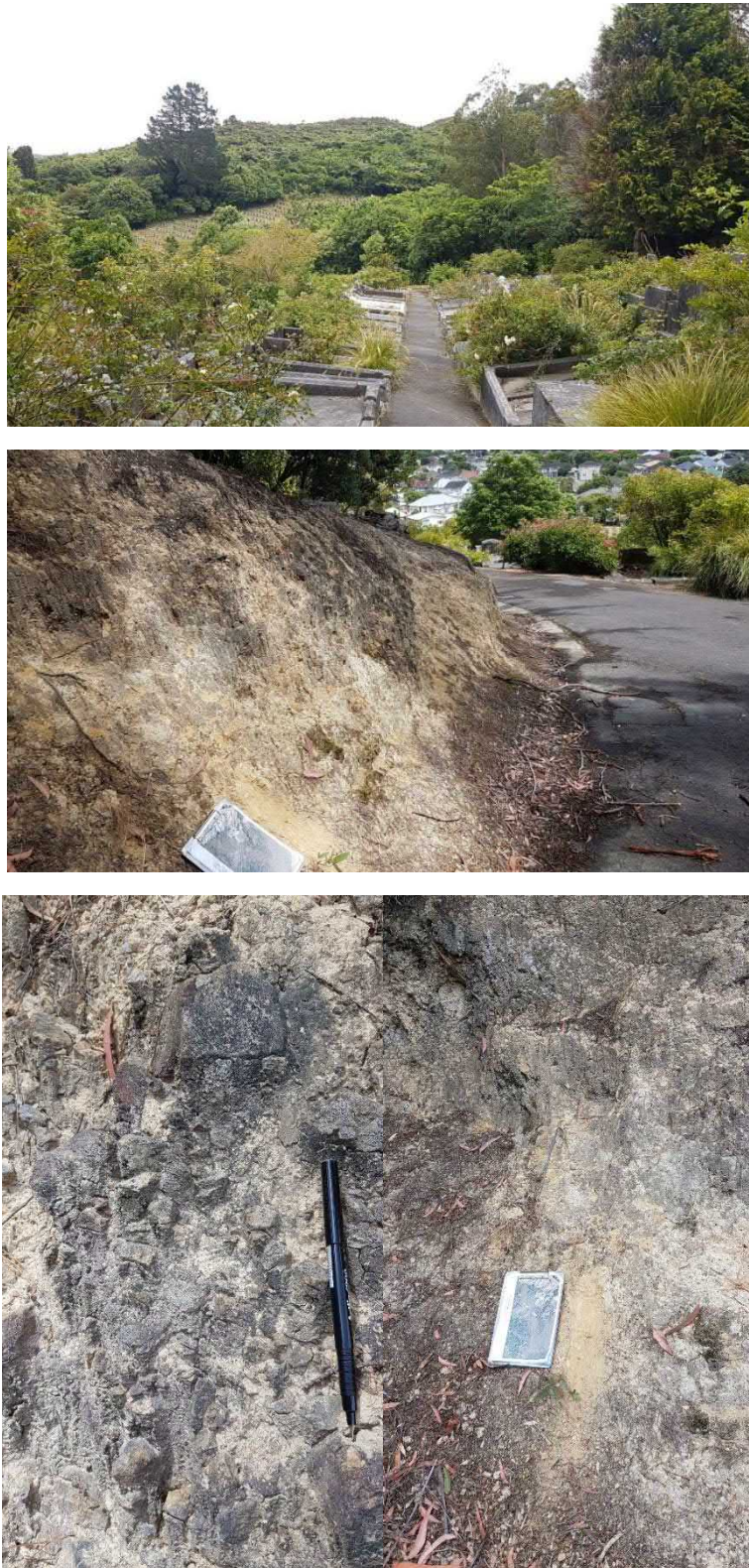
Figure B2 – Cambridge Terrace site photos: approximately 2m high cut slopes around the perimeter of the Taita cemetery 300m from the proposed reservoir site. Exposing completely weathered, greywacke rock.
