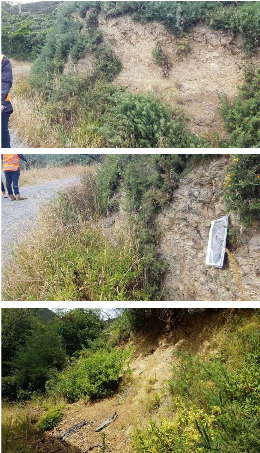
Figure B3 – Gracefield 2 site photos: approximately 2m high cut slope along the access track (top and middle photo) and 8m high cut slope around the perimeter of the existing reservoir (lower photo). Exposing highly weathered, greywacke rock.
