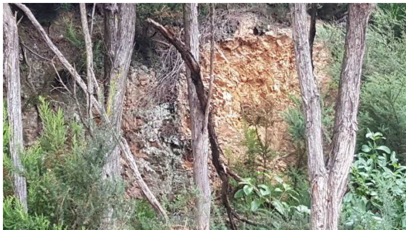
Figure B1 – Naenae 2 site photos: approximately 2m high slope cut adjacent to access track 100m from proposed reservoir site. Exposing highly weathered, highly fractured greywacke rock.
