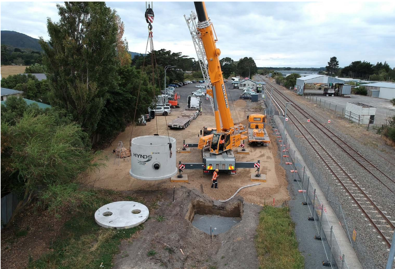
FIG. 5 18 module Up-Flo inside a 3.0m dia manhole treating a 6,500m 2 carpark at Featherston Railway station. Credit SDCL for image.
