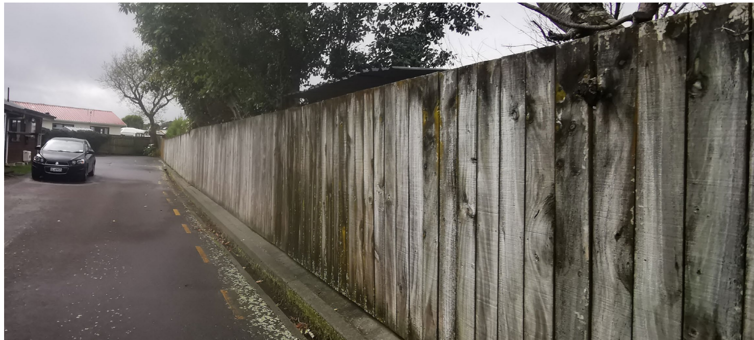
Existing southeastern boundary fence to be retained and waterblasted where in good condition. If damaged, replace with matching height vertical timber board fence.
