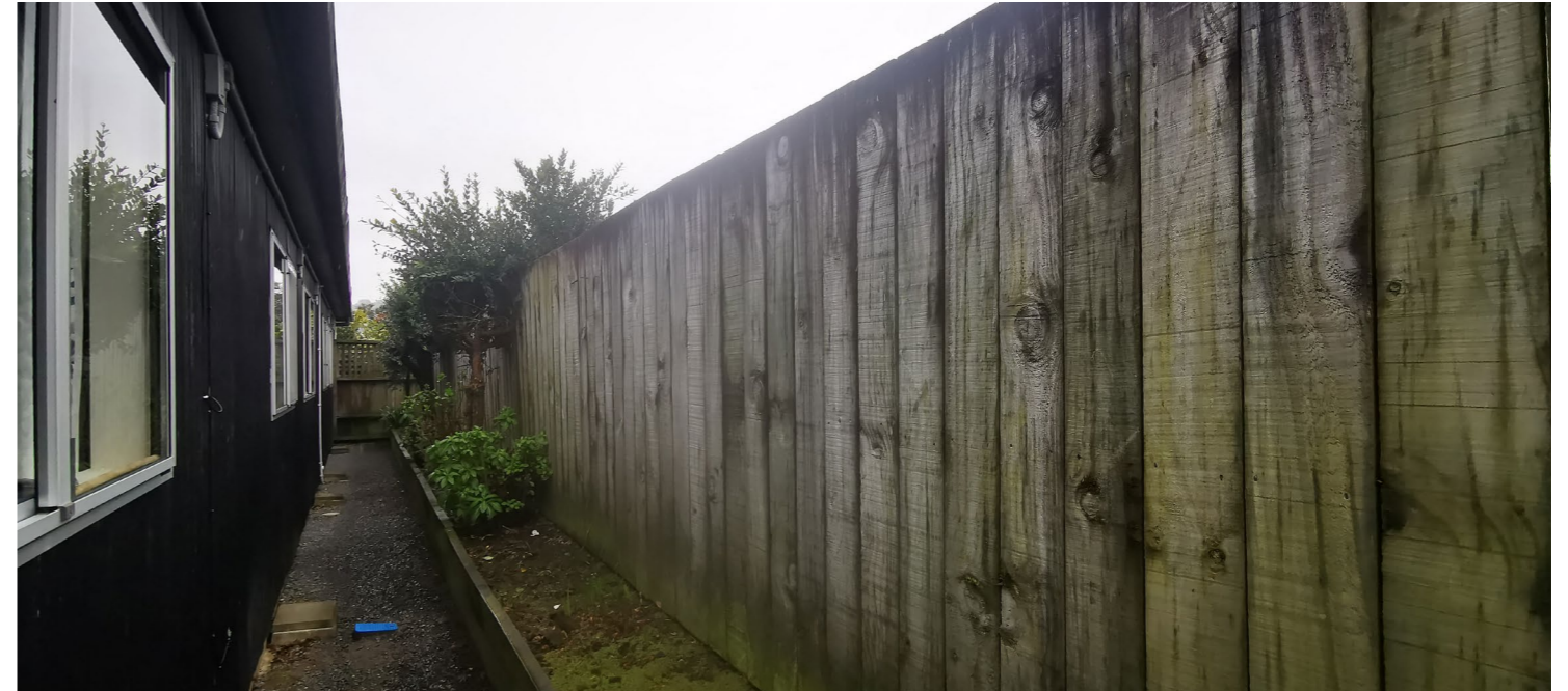
Existing northern boundary fence and retaining to be retained and waterblasted where in good condition. If damaged, replace with matching height vertical timber board fence.
