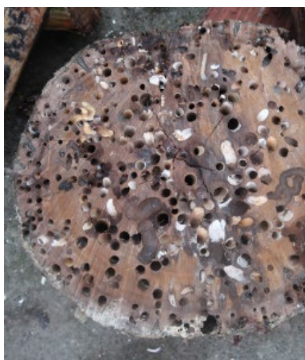
Figure 8: Marine borer damage to a section of pile removed from Petone wharf
