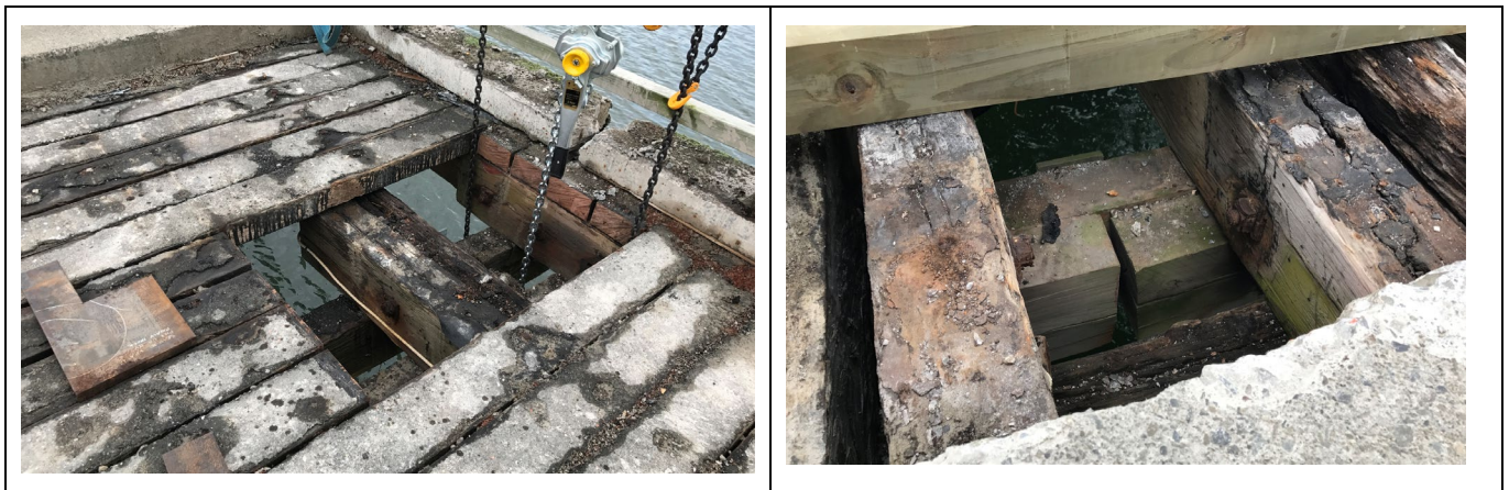
Figure 7: Exposed decking and stringer beams on Petone Wharf, note severe splits to exposed upper face of stringers.
