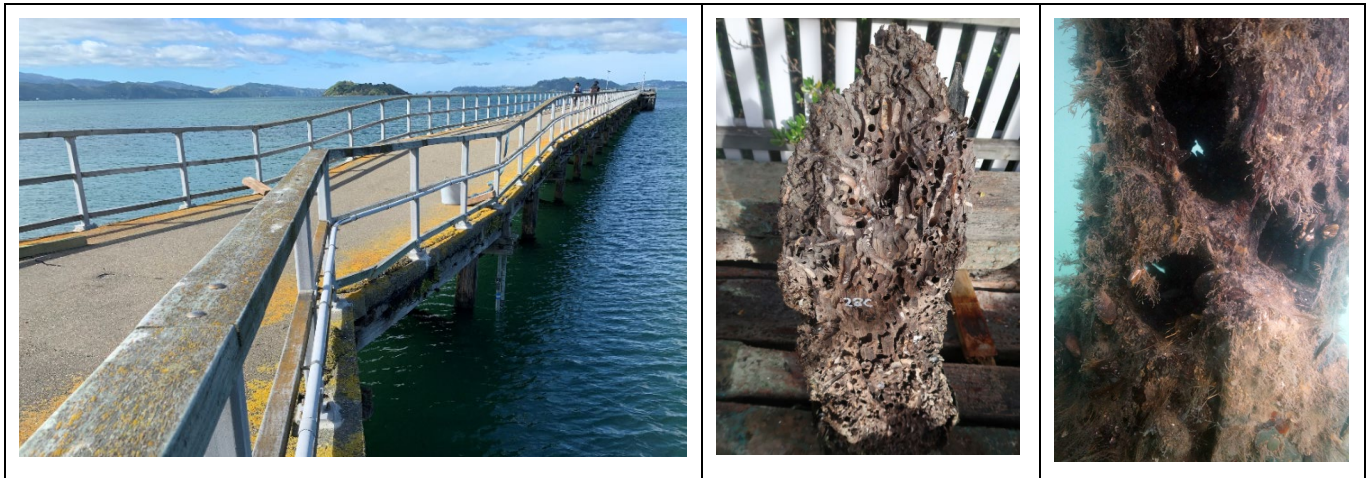
Figure 2 Dip in wharf deck over grid 28, and a length of the removed pile from this location showing severe deterioration from teredo worm. Worm damage to a pile on wharf head
