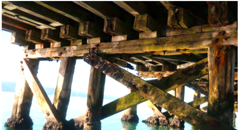
Figure 93. Timber packing between lowered cap beam and stringers. Source: Tom Arthur, Calibre Consulting Ltd., 2021 Wharf Condition Report, 25 June 2021.
