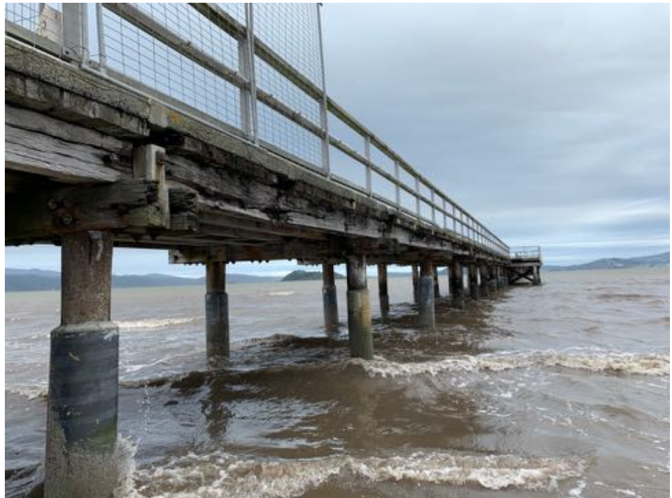
Figure 99. FRP Repairs on piles below the approach section of the wharf. Source: Calibre Consulting Ltd.
