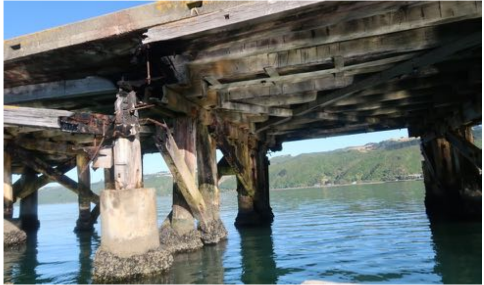
Figure 98. Fire damage to bent 63 on the head. Source: Calibre Consulting Ltd.
