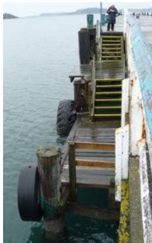
Figure 89. The previous timber access platform in 2012 prior to demolition. Source: Calibre Consulting Ltd.
