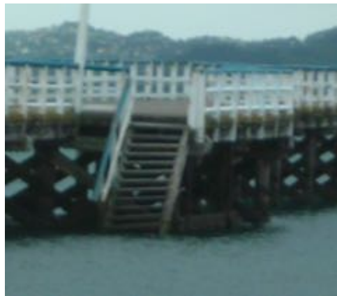
Figure 74. View of the cart refuge with stairs present, 2009. Source: Calibre Consulting Ltd., 2009
