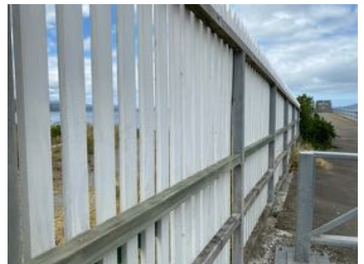
Figure 62. The current fence structure with metal stanchions and timber horizontals to match the current balustrade
