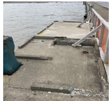
Figure 86. The Petone Wharf, November 2021, with the building removed and concrete foundations visible. Source: Calibre Consulting Ltd.
