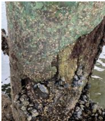
Figure 102. Some remaining copper sheathing on a pile. Source: Calibre Consulting Ltd.
