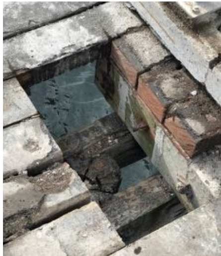
Figure 71. The timber decking below the concrete topping on the approach exposed during a test. Source: Calibre Consulting Ltd.
