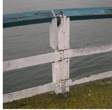
Figure 66. The handrail as of 2021 with multiple repairs. The toprail and post are as per the original specification, however the base and mid rails may have been replaced. Source: Calibre Consulting Ltd.
