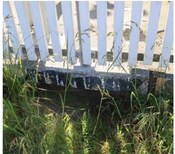
Figure 72. The edge of the concrete wharf deck on the entrance above the sand dunes. Source: Calibre Consulting Ltd.
