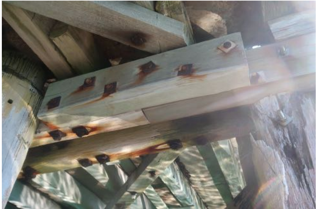
Figure 101. Repaired/replaced cap beam below the head constructed largely from new timber in original configuration. Source: Calibre Consulting Ltd.
