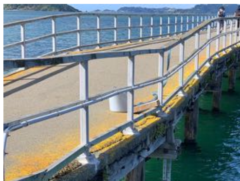
Figure 63. Current metal and timber balustrade over slumped portion of the approach. Source: Calibre Consulting Ltd.
