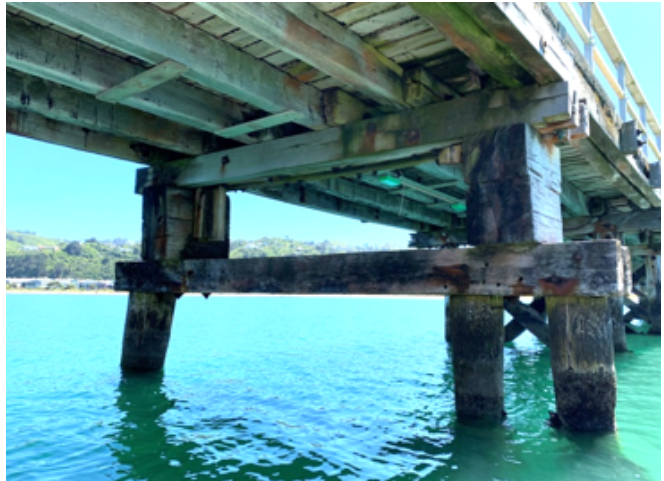
Figure 95. Bent 46 with timber blocking between upper and lower pile caps. Note the missing original pile on the left-hand side with the top of the original pile still in place.
