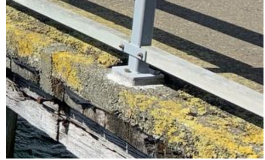
Figure 70. Side view of the concrete decking on the approach over the original timber decking. Source: Calibre Consulting Ltd
