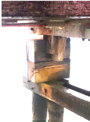
Figure 94. Timber blocks between upper and lower pile caps on bent 45. Photo by Calibre Engineering.
