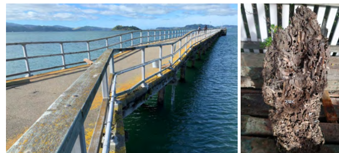
Figure 4 Dip in wharf deck over grid 28, and a length of the removed pile from this location showing severe deterioration from teredo worm
