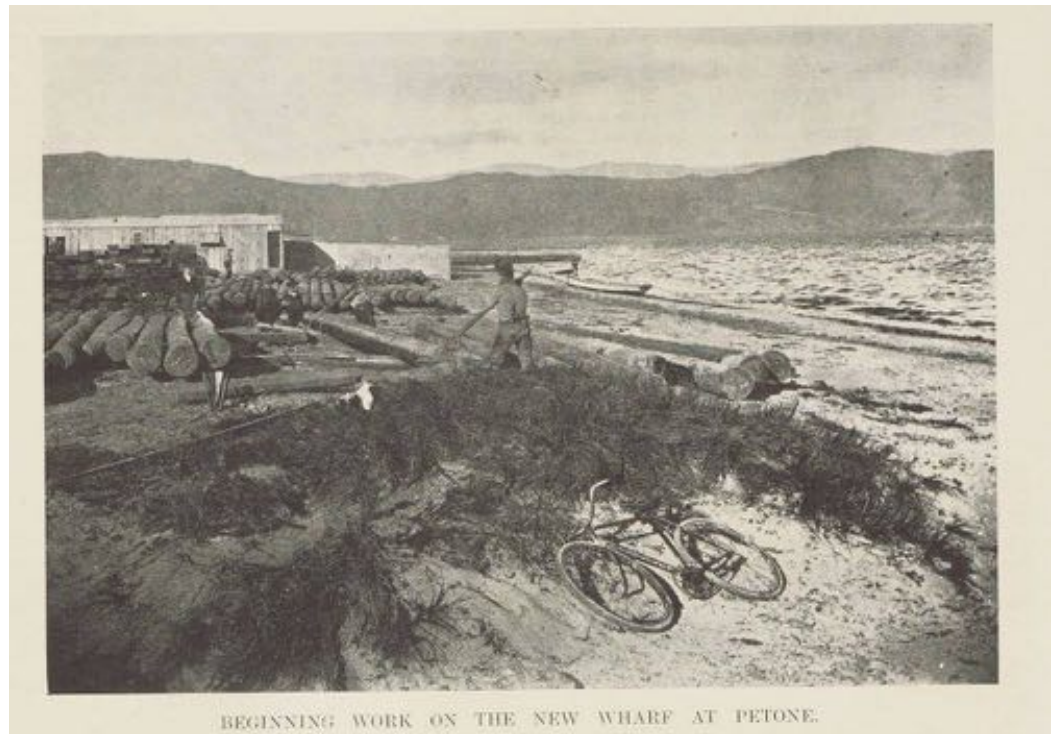
Figure 17. 1908 construction work on the Petone Wharf. Source: Sir George Grey Special Collections Auckland Libraries, NZG-19080624-37-1
