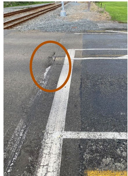
Figure 3-11: Minor Defects Circled
