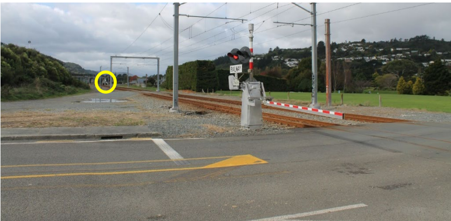
Figure 3-6: FLBs, HABs in Operation, Circle Shows Train at the Manor Park Station
