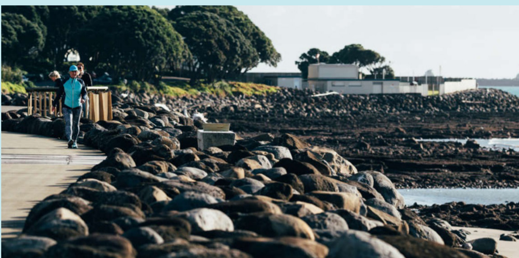
An example of rock revetment used on the New Plymouth coastal walkway
