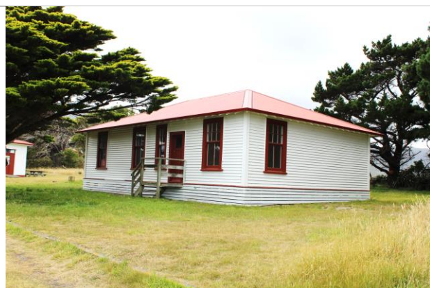
Figure 11: One of the 'keepers cottages, restored by the Friends of Baring Head conservation group.
