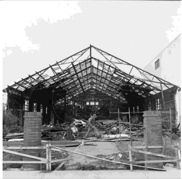
Figure 16: Demolition of the Horticultural Hall in 1958 after fire damage. Source: ATL, ID: EP/1958/0128-F
