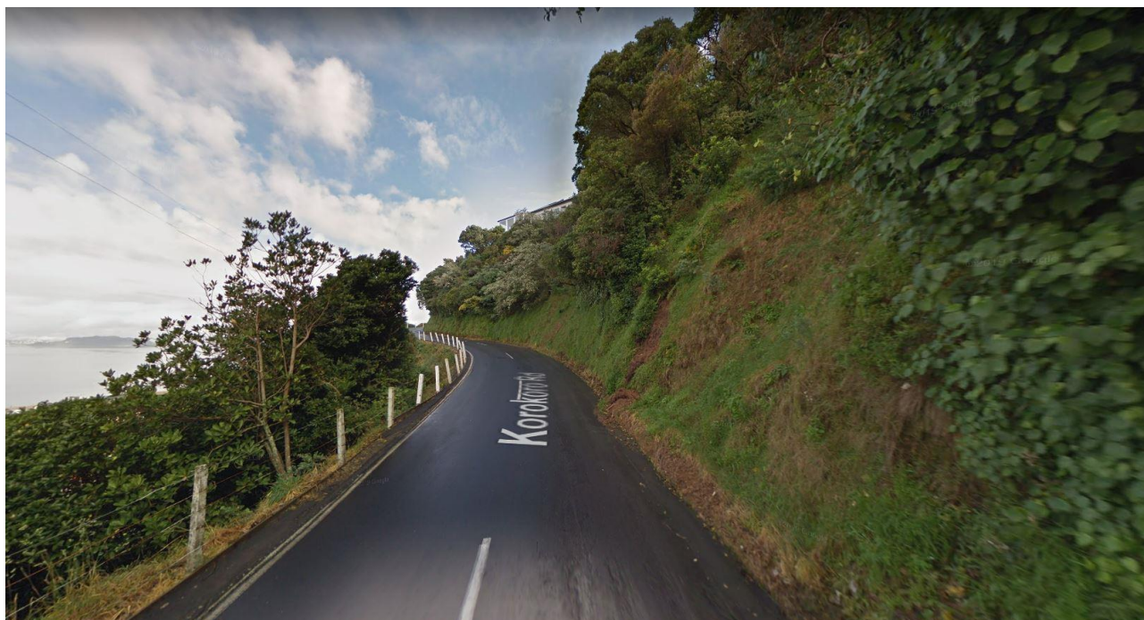
Figure 4: Korokoro Road, with steep cut slopes to the right of the road, and houses positioned behind the crest of these slopes. (Image from Google Maps Street View).
