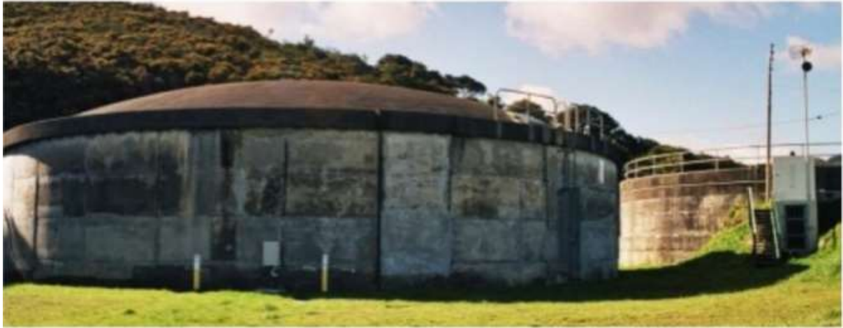
Figure 13 Point Howard Water Supply Reservoirs
