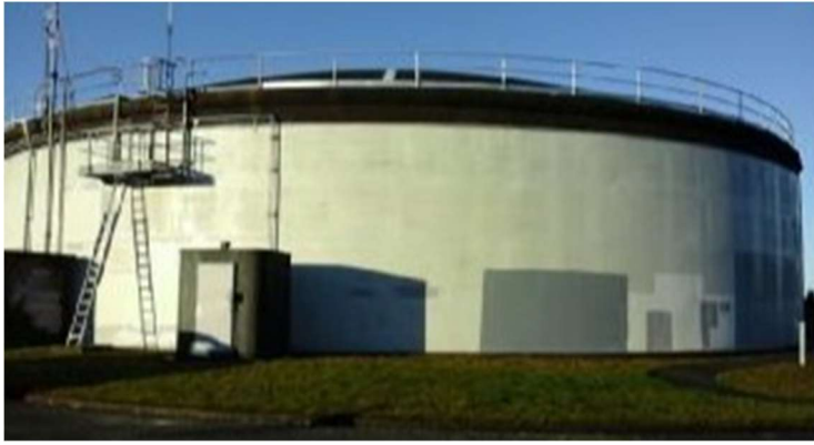
Figure 11 Maungaraki water supply reservoir
