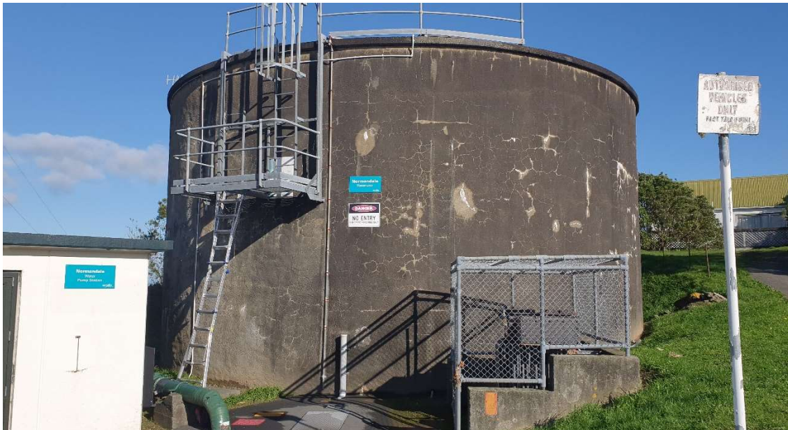
Figure 12 Normandale water supply reservoir
