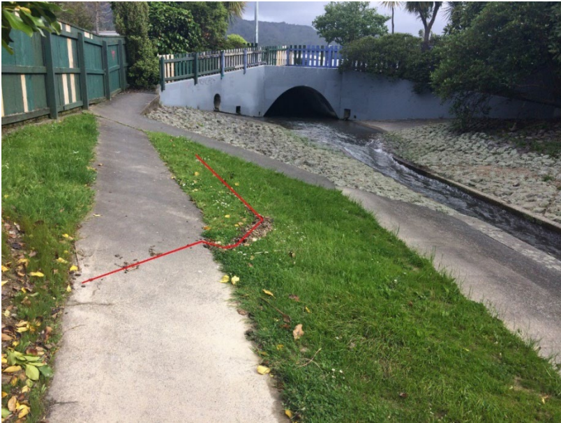
Figure 4-43: Outlet of Evans Street Arch following the 15 November 2016 rainfall event.
