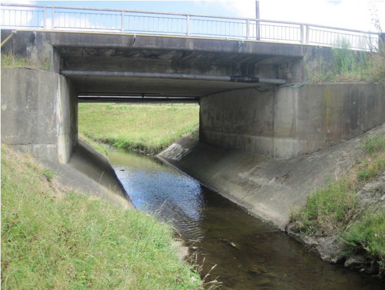
Figure 3-9: The Eastern Hutt Road bridge, represented in the model as a culvert.
