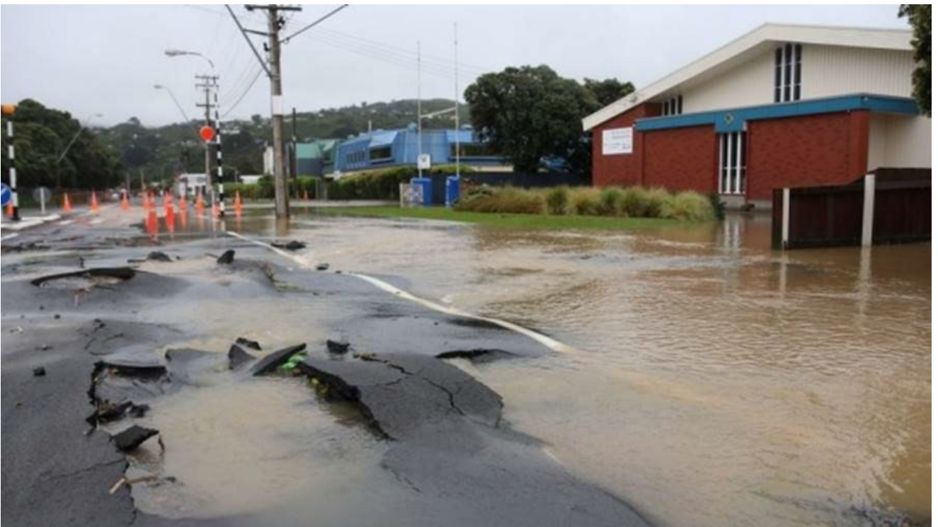
Figure 2-8 Road damage from the Western Hills gravity pressure main (15 November 2016).
