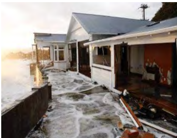
Figure 4: Beauchamp Cottage after storm damage, 2013. Source: Satbhagat R. Bettoni
