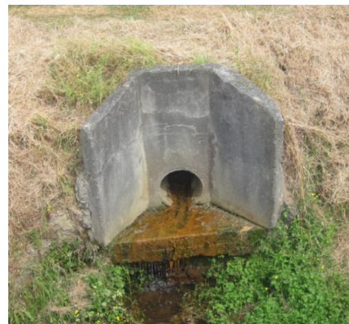
Figure 4-9: Outlet with concrete apron and weir
