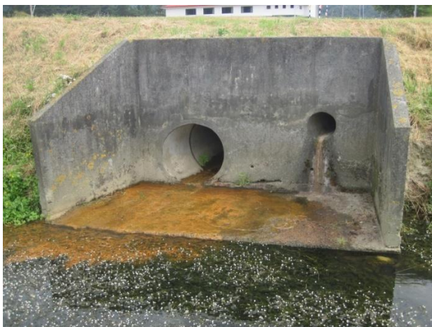
Figure 4-8: Outlet with concrete apron and weir
