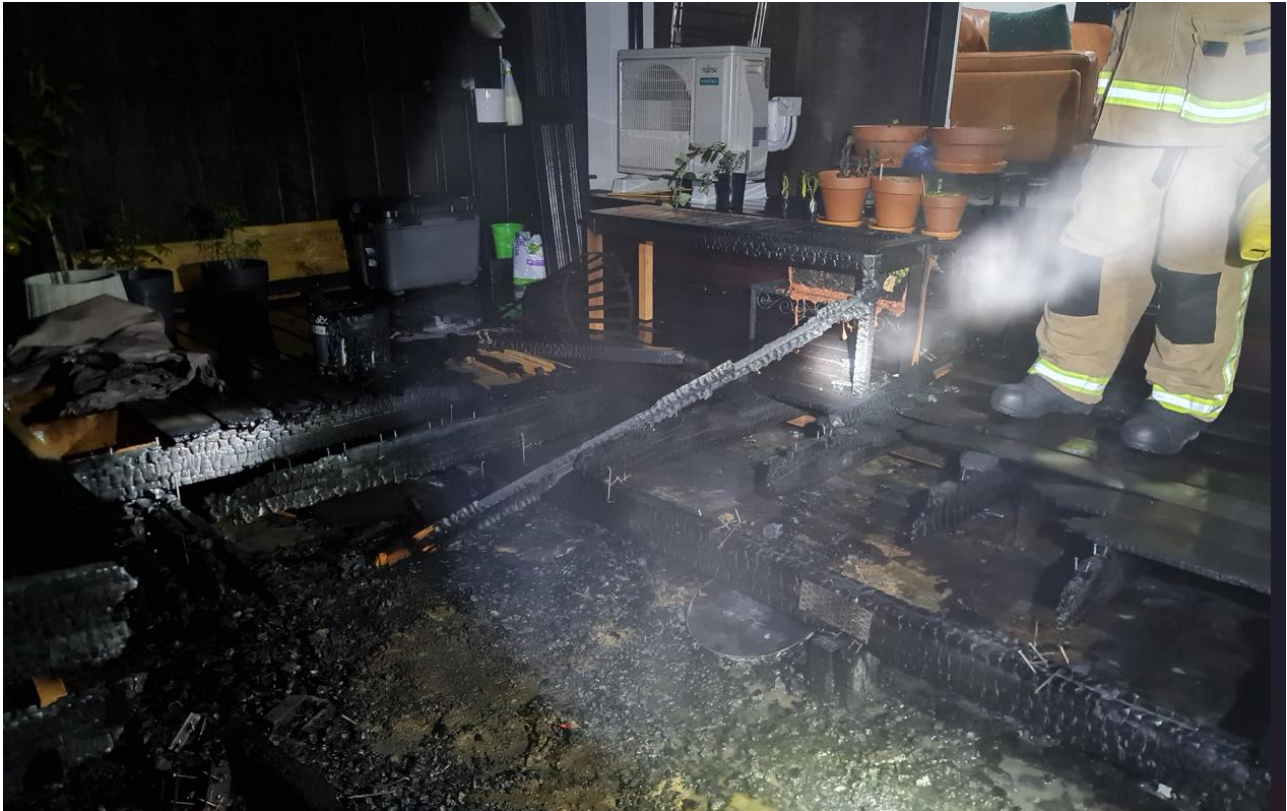
Figure 10: Damage to the unit 19 deck and contents.
