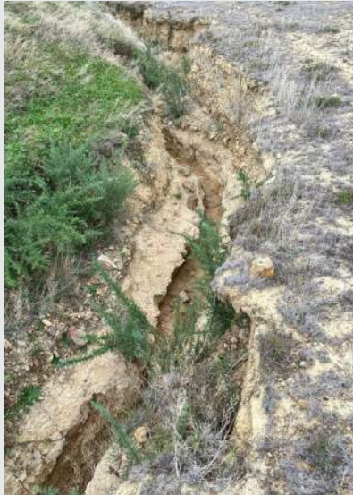
Erosion shown in drainage channel.
