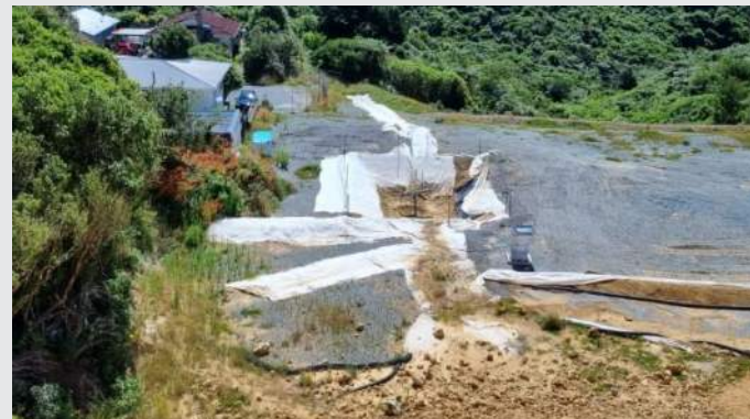
Sediment detention pond at base of EW 05
