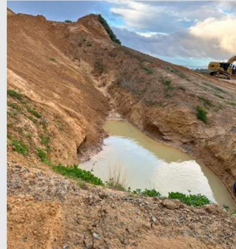
Stormwater control, possible blocked culvert
