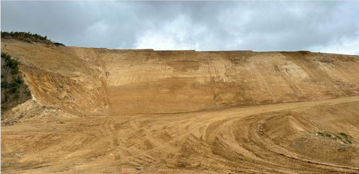
EW02 - minor slip visible at the top.
