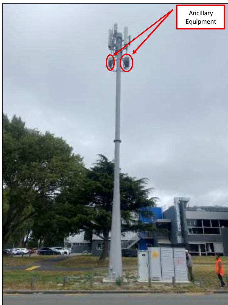
Figure 1: Mobile Phone Facility identifying ancillary equipment
