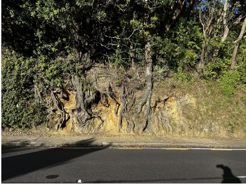
Figure 4. Gravel overlying weathered greywacke below 12 Park Road.
