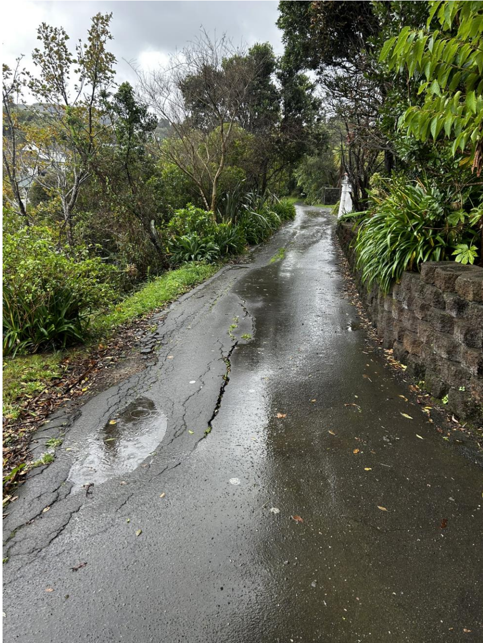
Figure 7. Tension cracks disrupting sealed upper carriageway.
