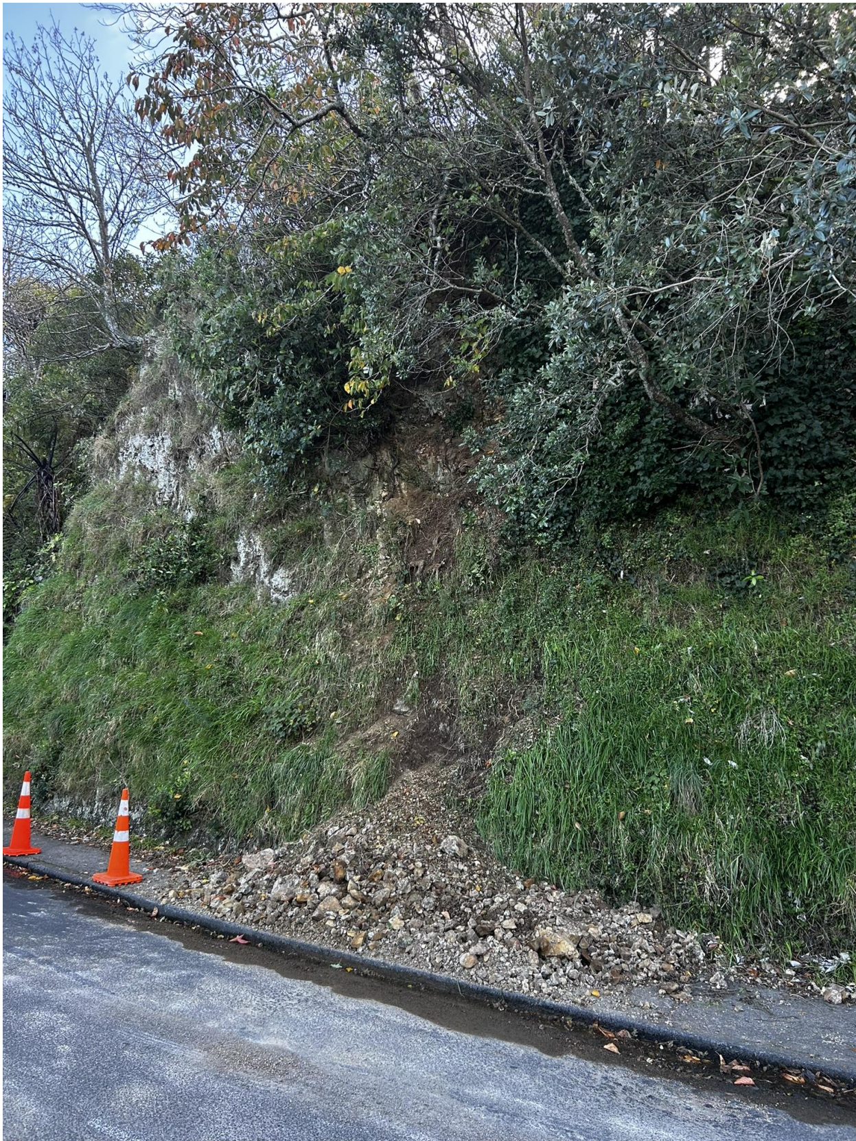
Figure 10. Rock fall from slope below 10 Park Road, debris covering pedestrian footpath.
