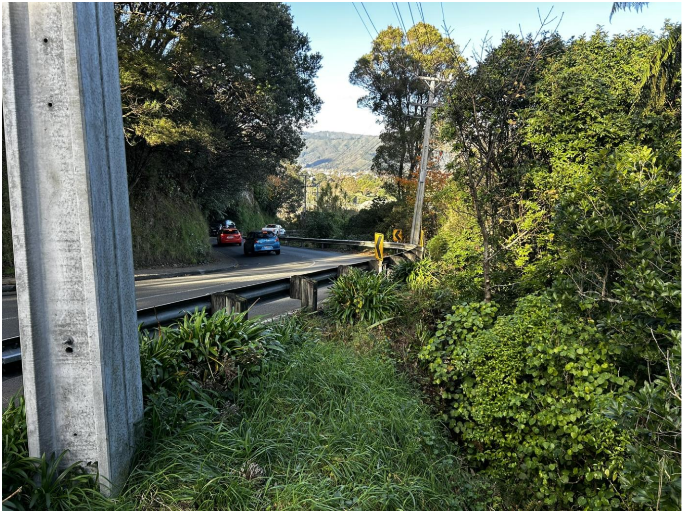
Figure 11. Slope below 12A Park Road showing lean on power pole.
