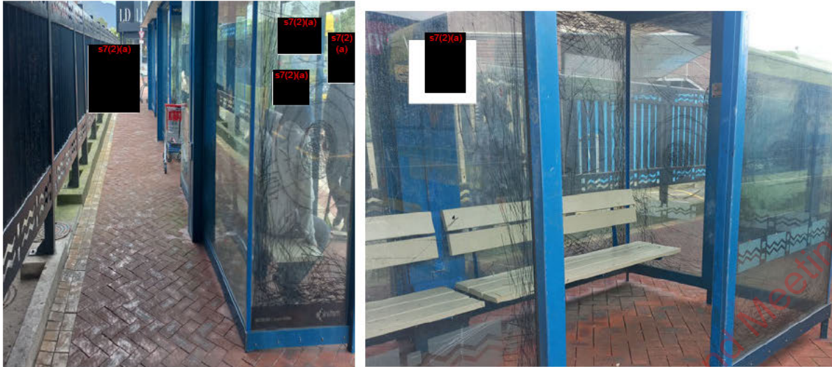
Bus Shelter – Glass replaced (Hit with a hammer / Youth) / Graffiti
