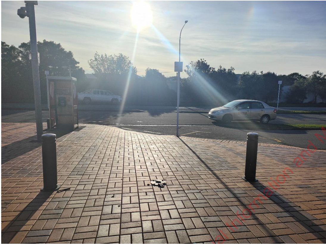
Ref 5 Bollard missing outside the Naenae Library
