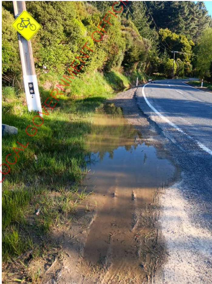
Figure 9: Flooding from 915 Wetlands
