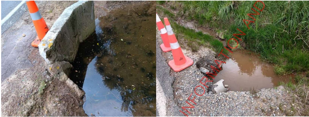
Figure 8: Blocked culverts going under Coast Road
