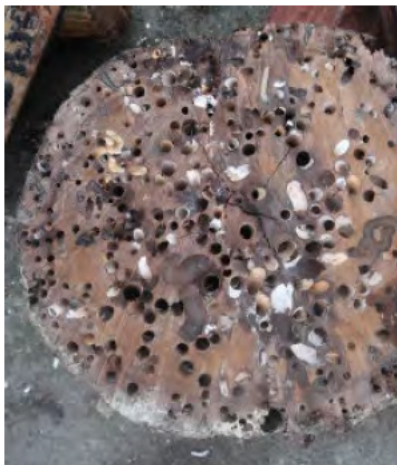
Figure 8: Marine borer damage to a section of pile removed from Petone wharf
