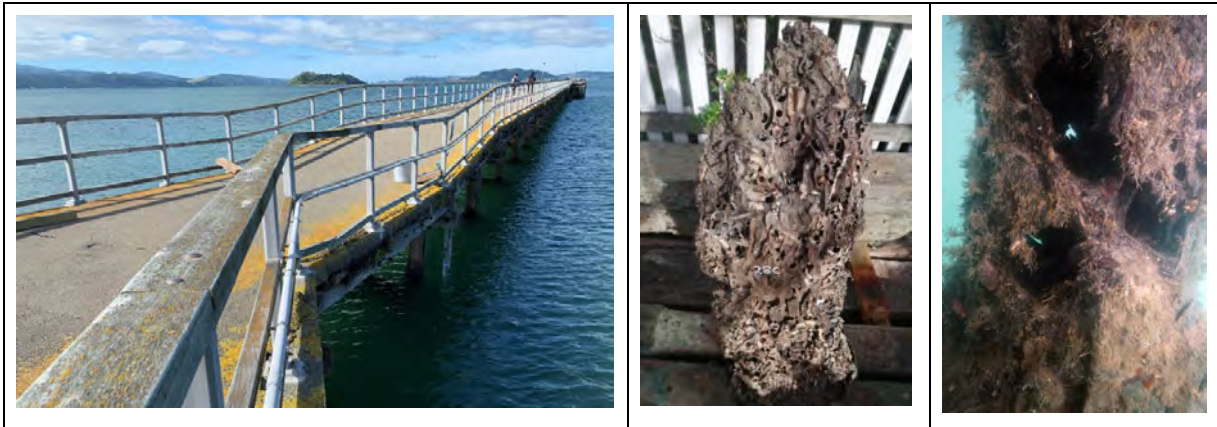
Figure 2 Dip in wharf deck over grid 28, and a length of the removed pile from this location showing severe deterioration from teredo worm. Worm damage to a pile on wharf head
