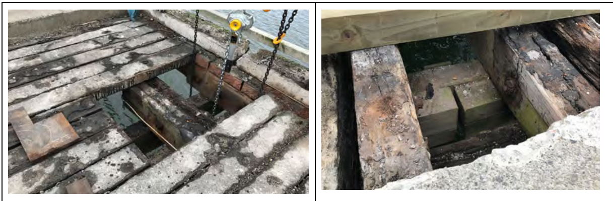
Figure 7: Exposed decking and stringer beams on Petone Wharf, note severe splits to exposed upper face of stringers.
