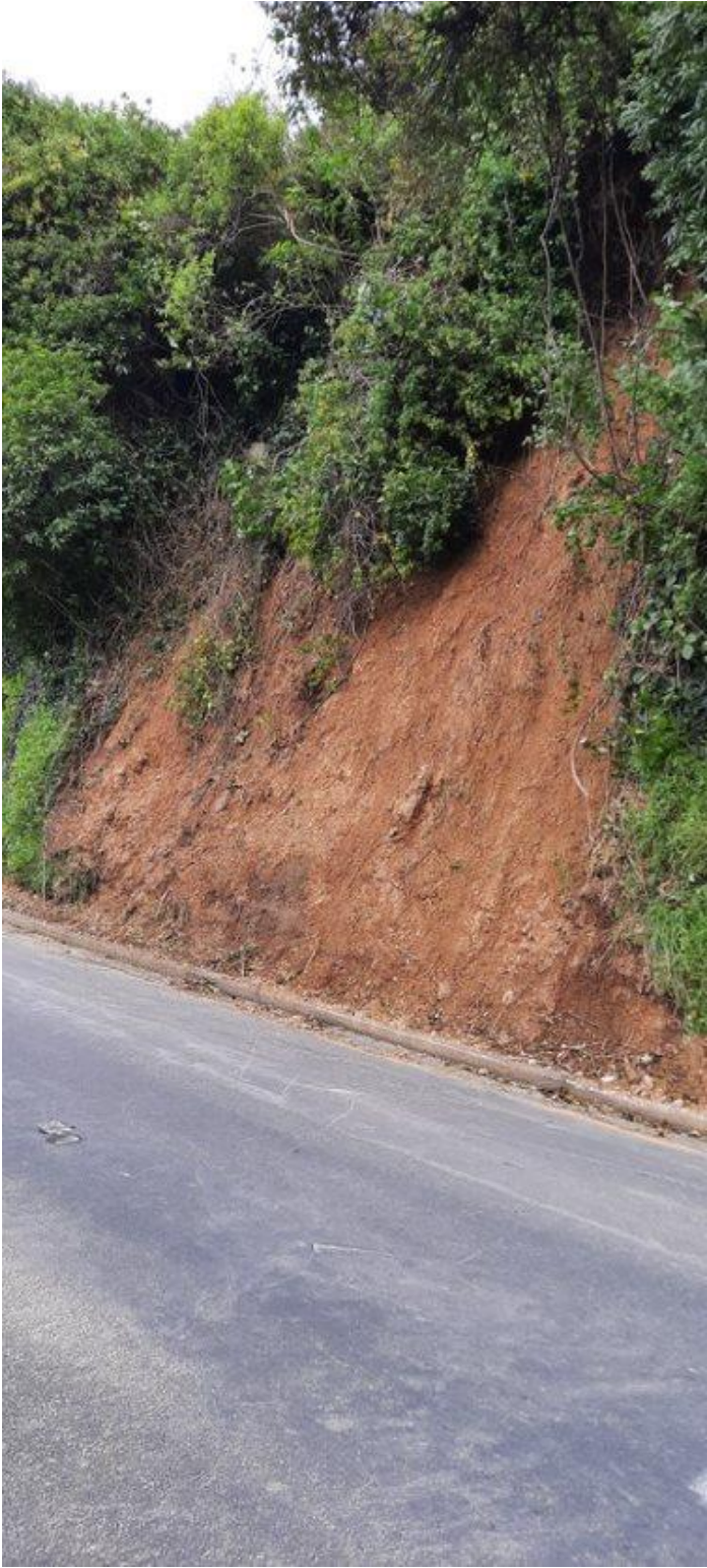
Minor slip along Korokoro Road 1, 2022
