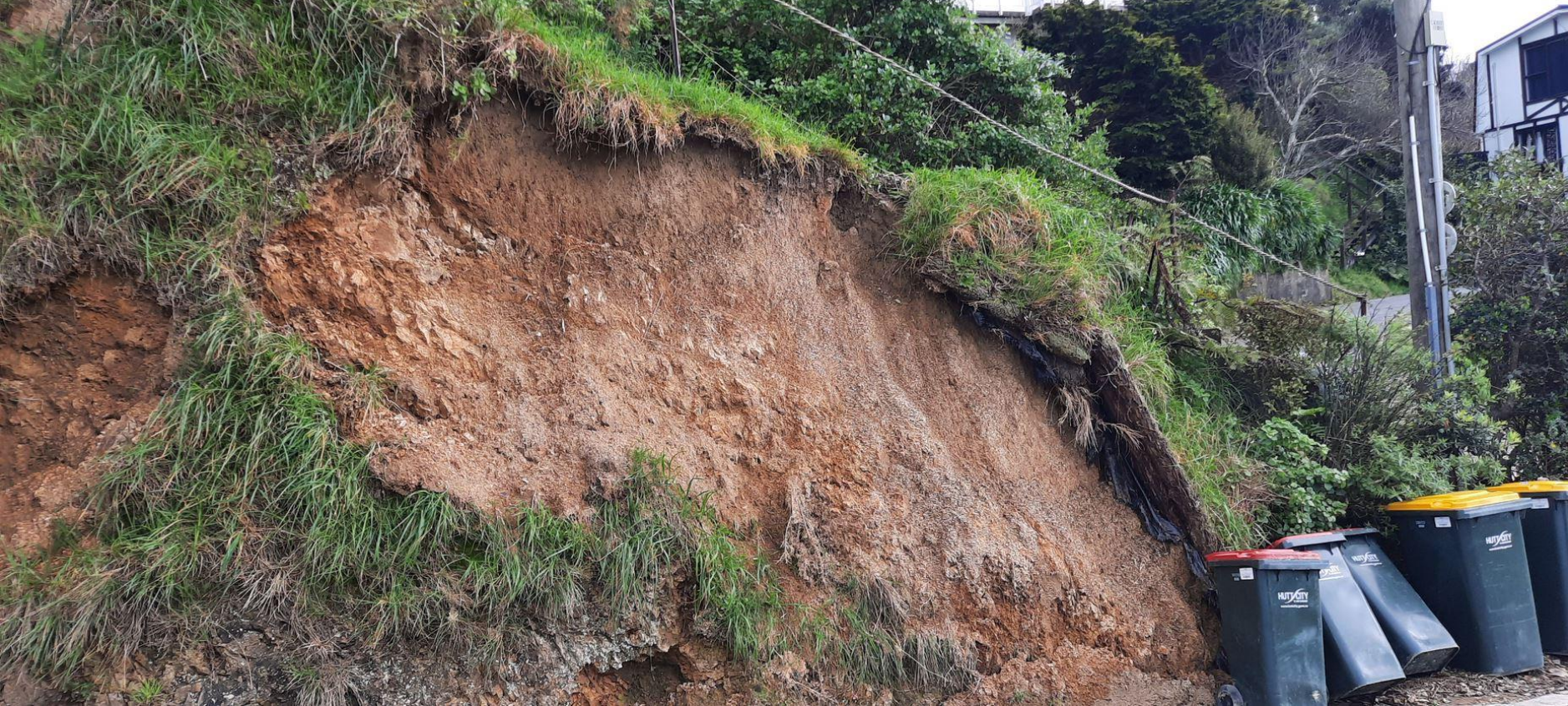
Minor slip under concrete steps along Korokoro Rd, 2022
