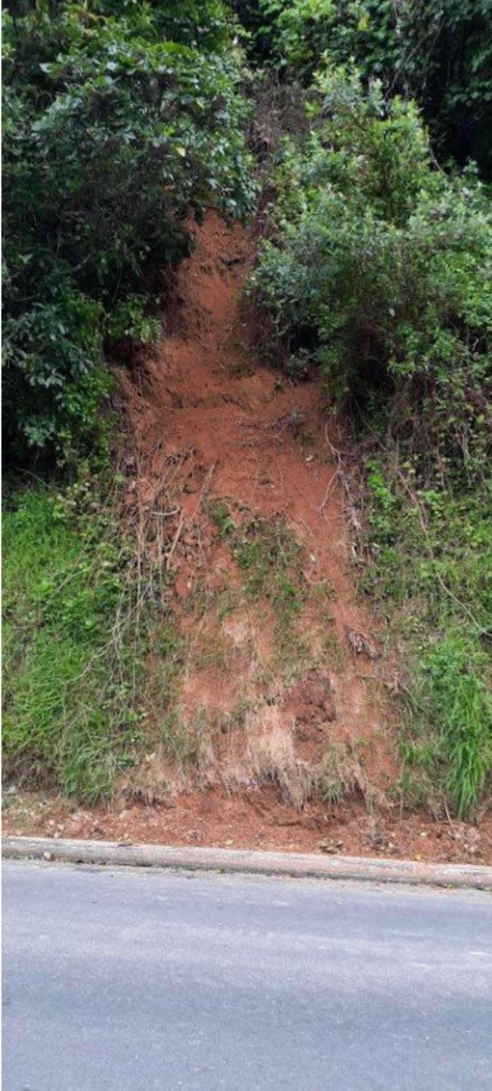
Minor slip along Korokoro Road 2, 2022
