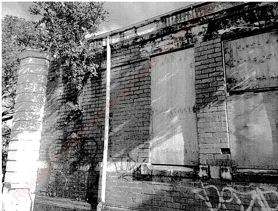
Figure 5 East wall of Old Court House with horizontal crack through concrete lintel
