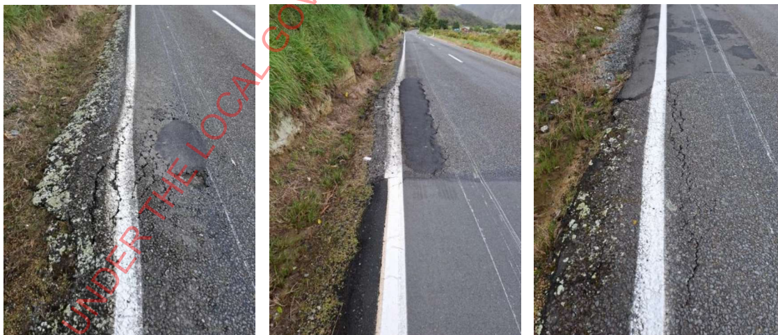
Examples on the Coast Rd of soft edges collapsing
