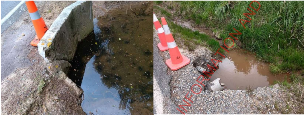
Figure 8: Blocked culverts going under Coast Road
