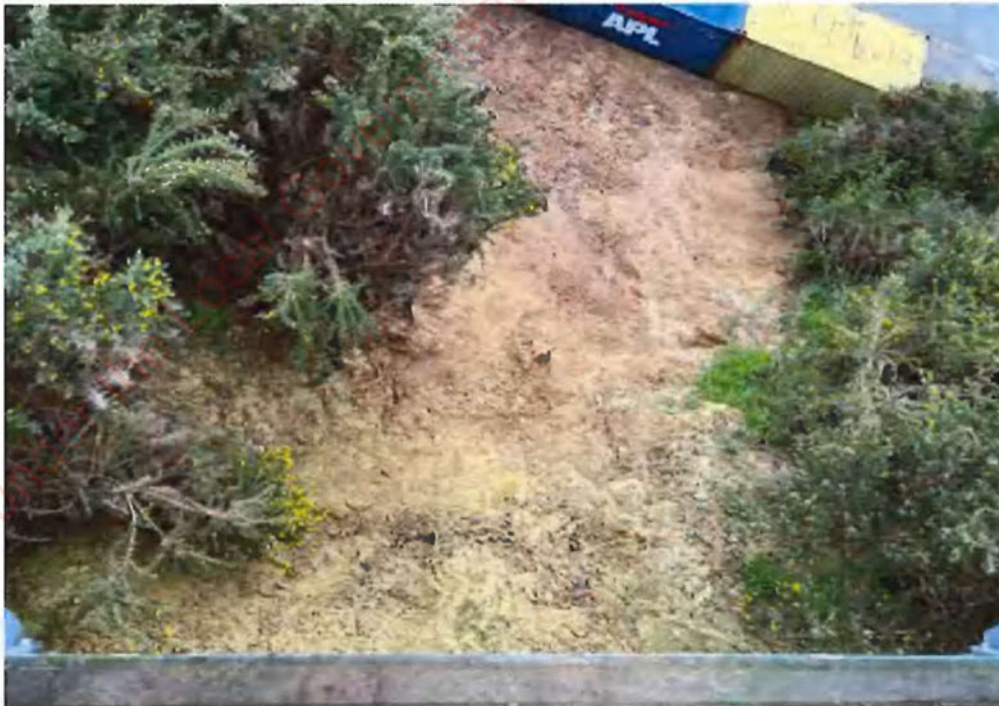
Photograph 4: View of landslip 1 from above – taken from deck (Comparison photo taken 26 July 2022).
