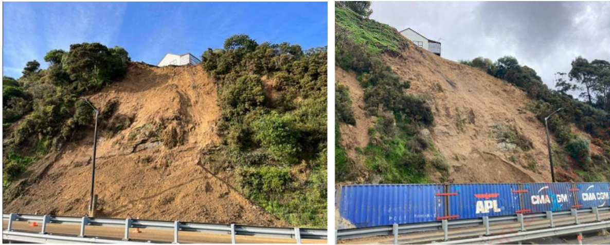
Figure 1 Left: Initial slip (21 July 2022). Right: Current slope condition following temporary works (14 September 2022)
