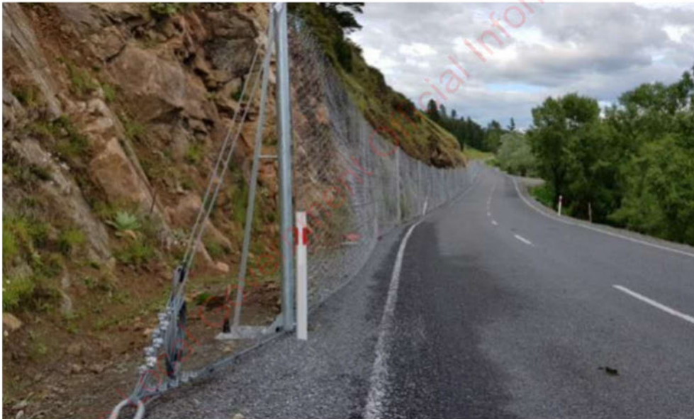
Figure 8 Example of a roadside catch fence
