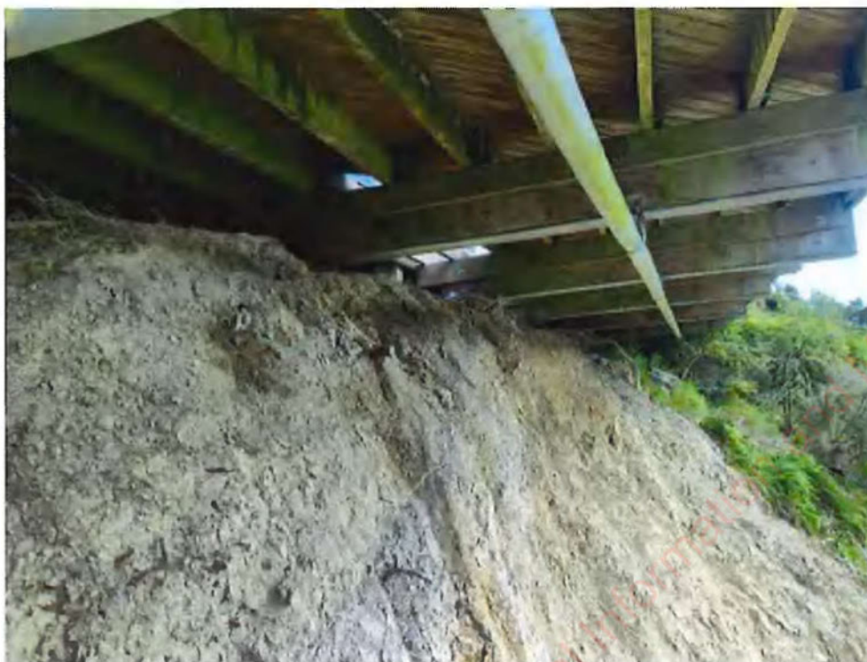
Photograph 17: View at top of landslip 1 from below deck (looking from east to west) after trimming/clearing of slope (Photo taken 15 September 2022).
