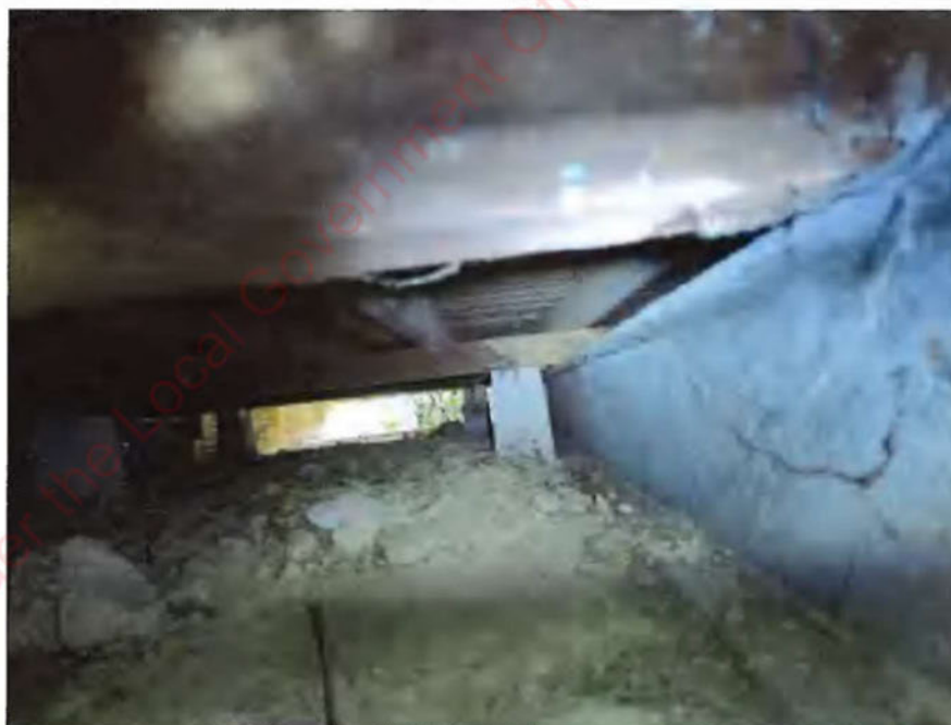
Photograph 16: View through internal floorboards of dwelling looking at concrete pile dwelling foundations and separate steel cantilevered beams for deck (Photo taken 11 August 2022).
