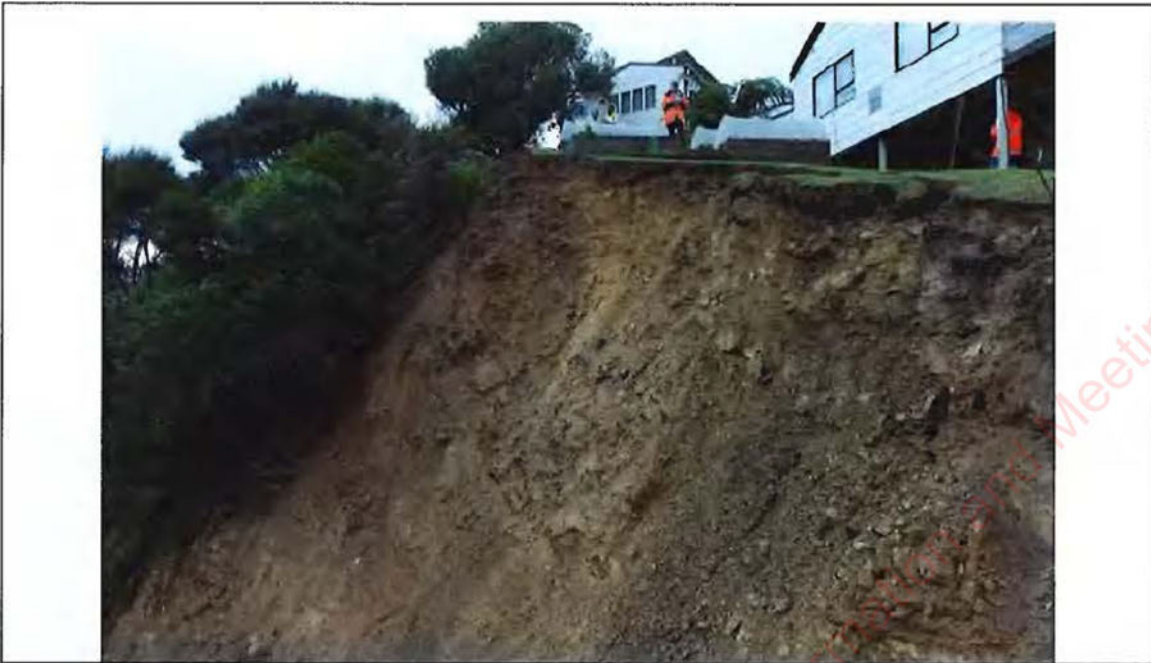
Photograph 7: View facing up to the east, showing landslip headscarp and material. Taken 26 July 2022.
