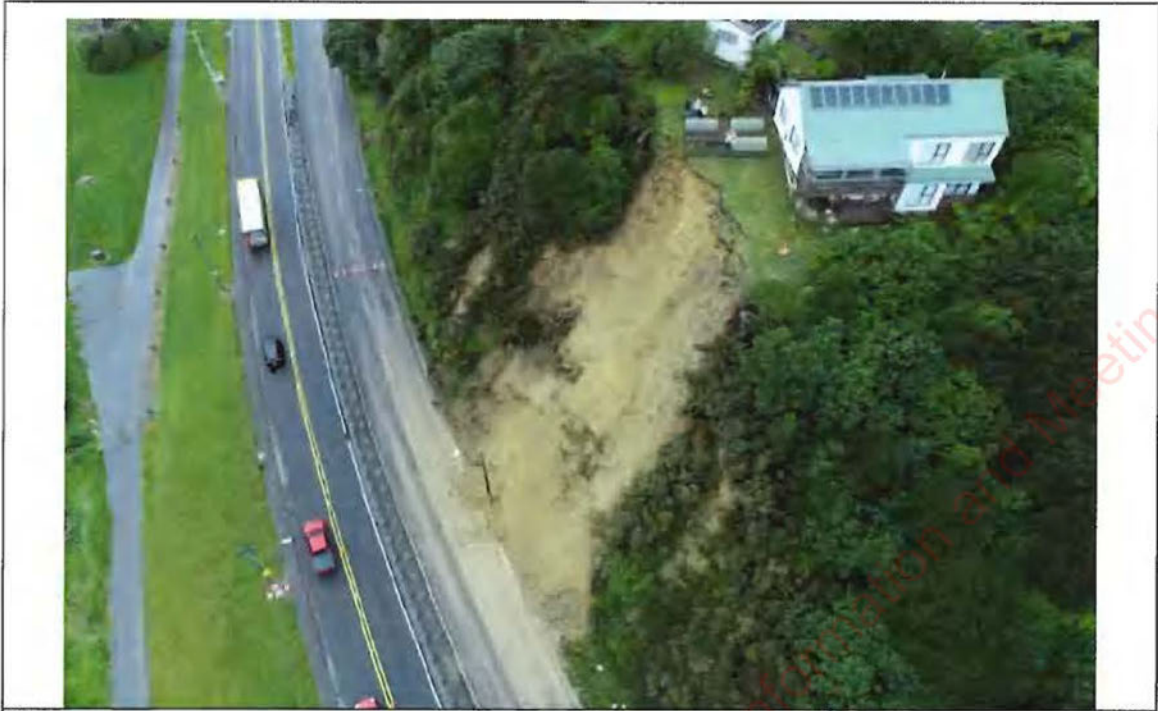
Photograph 5: View facing east from above, showing entire landslide. Taken 26 July 2022.
