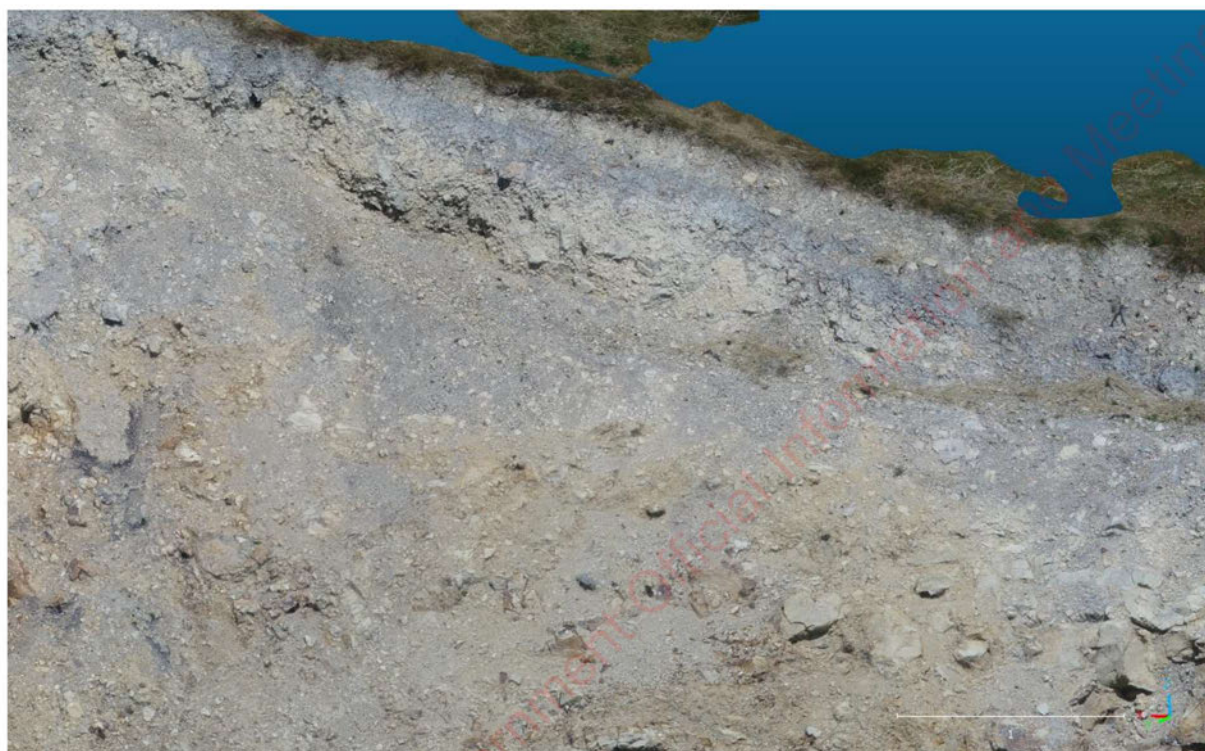
Figure 4 Colluvium exposed at top of slope
