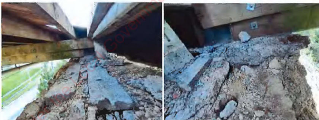
Photograph 18: View under deck looking at foundations after trimming/clearing of slope for Landslip 1 (Photo taken 15 September 2022).
