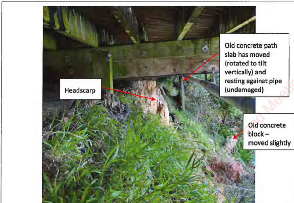
Photograph 7: View at top of landslide 1 from below deck (looking from east to west) (Comparison photo taken 26 July 2022).
