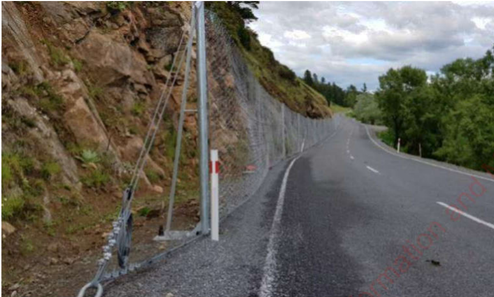
Figure 8 Example of a roadside catch fence
