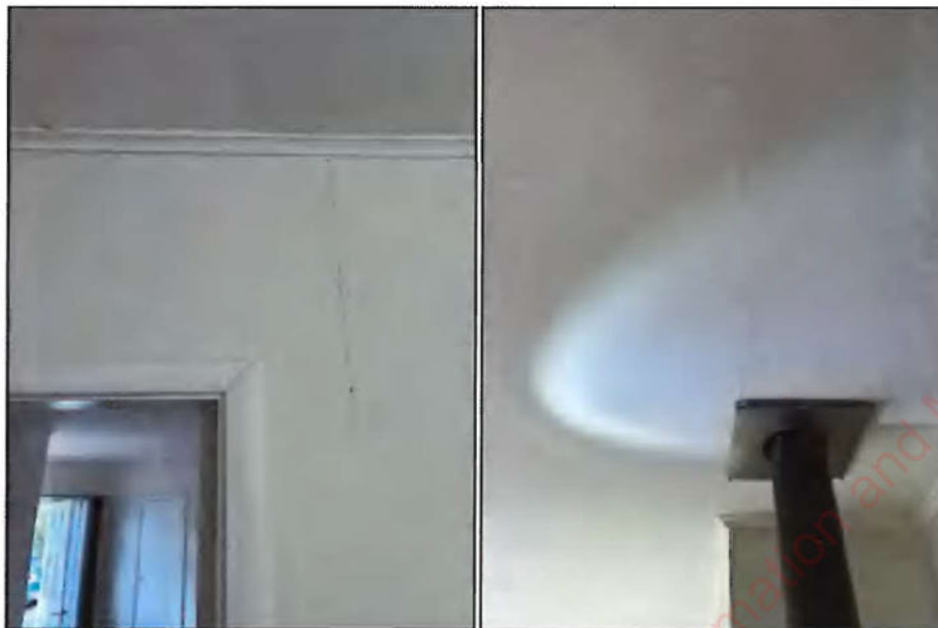
Photograph 15: Internal cosmetic cracking damage to internal walls in approximate centre of dwelling as a result of relaxation of land from behind the headscarp of landslip 1 (Photo taken 11 August 2022).
