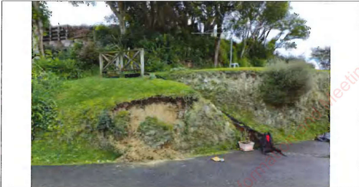
Photograph 19: Landslip 2 within 8 m of clothesline above accessway. View looking north-west (Photo taken 26 July 2022).
