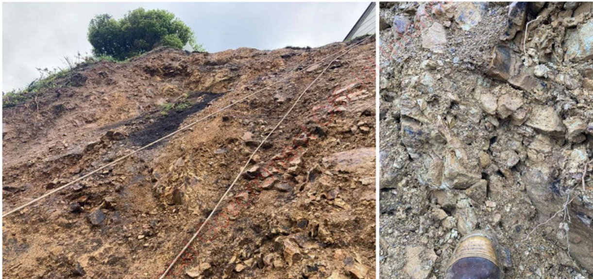
Figure 2 Dilated rock mass and loose colluvium ravelling from the upper reaches of the slope
