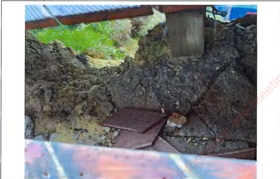
Photograph 11: View under undamaged deck (looking north) down the landslip 1 (Photo taken 26 July 2022). Note old timber pile is not attached to the deck (undamaged).
