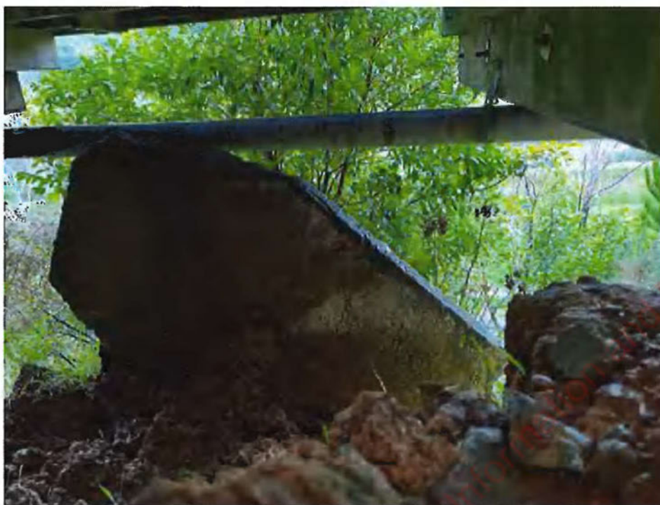
Photograph 9: View under deck (looking north) of landslip 1 (Photo taken 26 July 2022). Old concrete path slab has moved (rotated and tilted vertically) and resting against pipe (undamaged).
