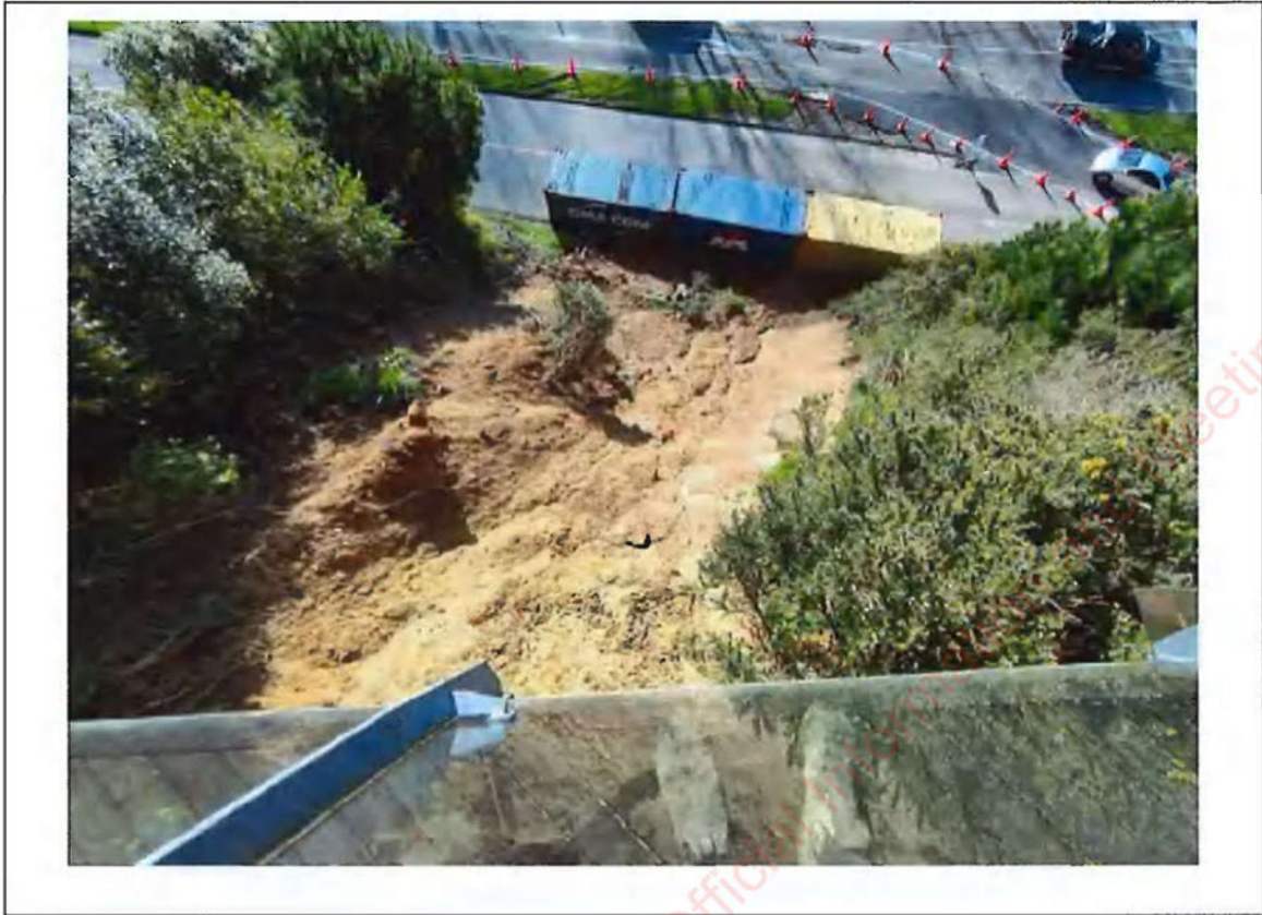
Photograph 5: View of landslip 1 from above – taken from deck (Comparison photo taken 23 August 2022).
