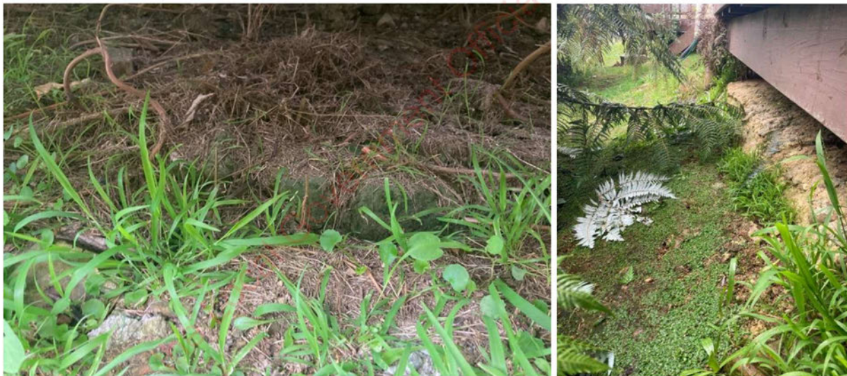
Figure 4 Left: Tension cracks along the western perimeter of the building. Right: ~200 mm of subsidence
