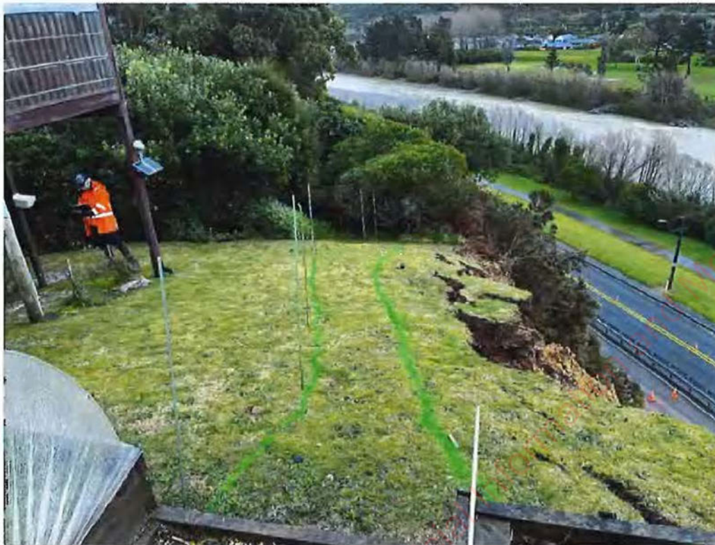
Photograph 3: View looking west along the length of the area behind the observed landslip headscarp. Taken 26 July 2022.
