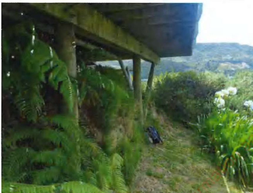
Photograph 13: Access to landslip 1. View from below eastern side of deck looking north-west (Photo taken 10 January 2022). This section of deck is supported by timber poles and timber beam.
