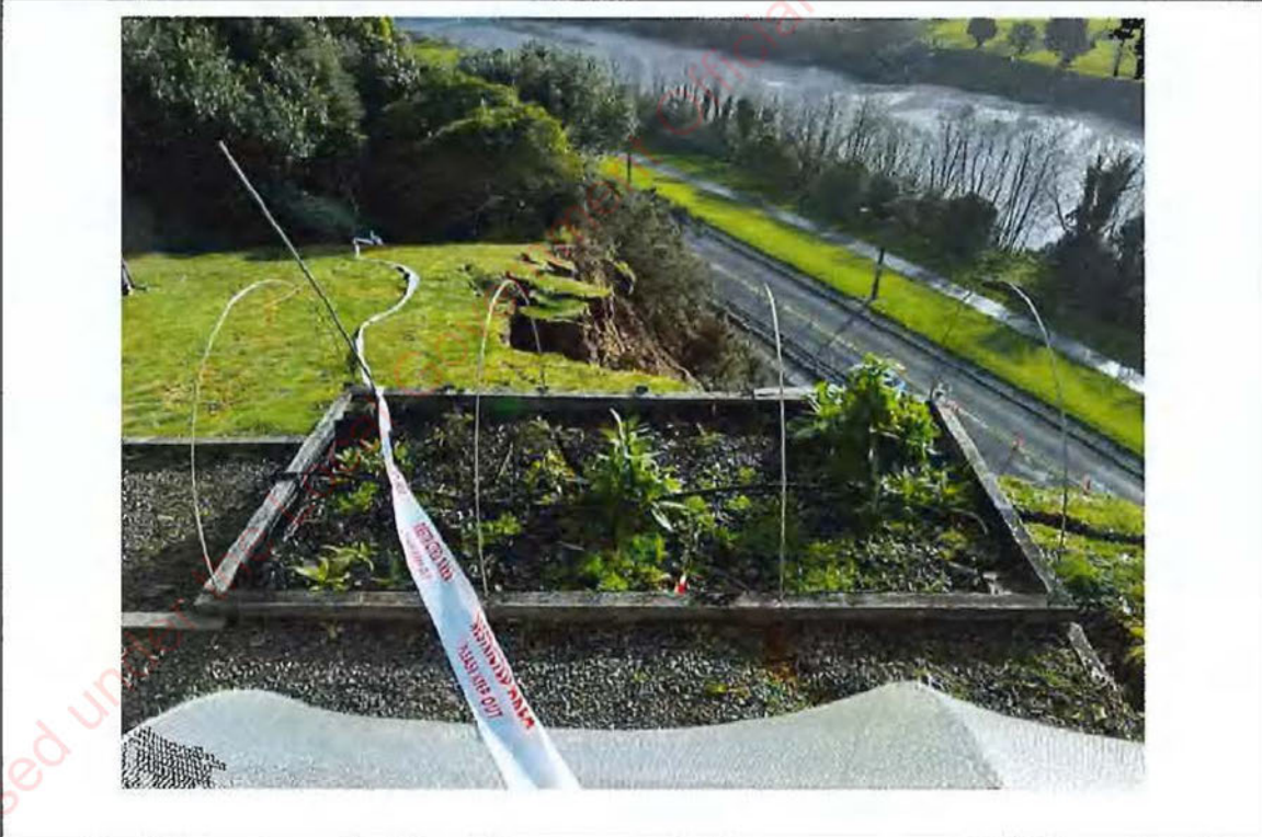
Photograph 8: View looking west along the length of the area behind the observed landslip headscarp. Taken 11 August 2022.
