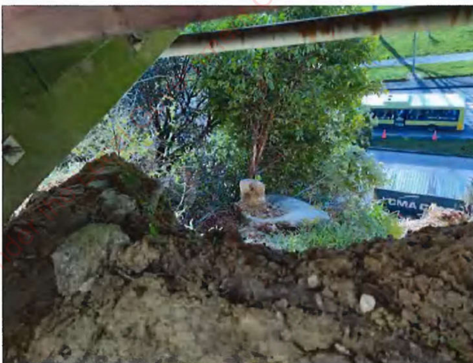
Photograph 10: View under deck (looking north) of landslip 1 (Photo taken 23 August 2022). Old concrete path slab has moved downslope as a result of further land movement.
