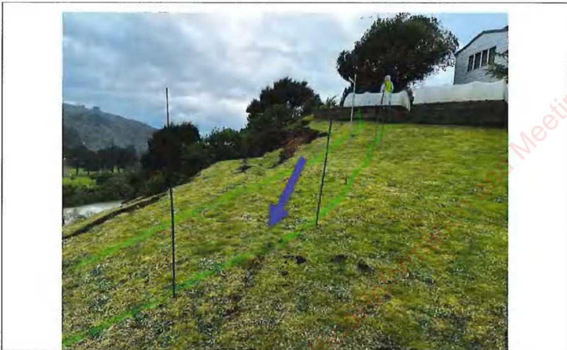
Photograph 1: View facing east from property, showing tension crack in the foreground (arrow). Taken 26 July 2022.
