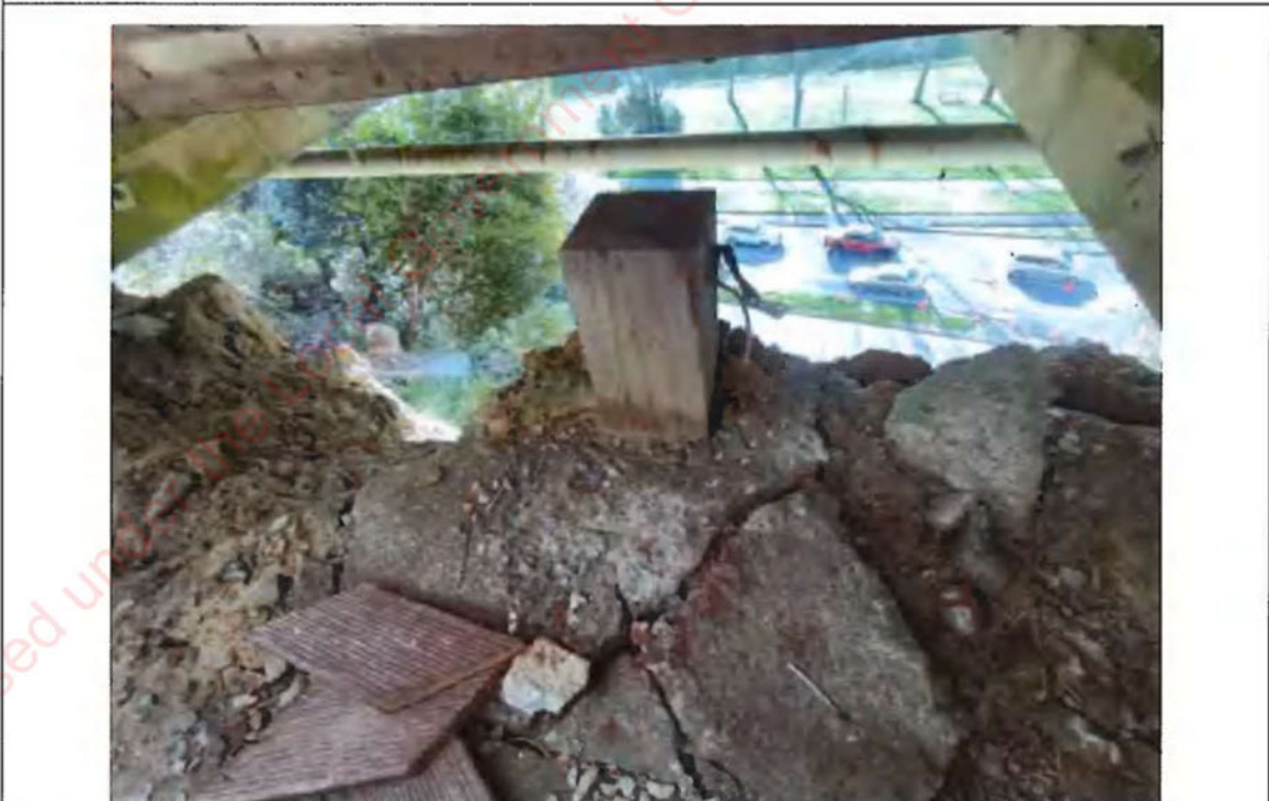
Photograph 12: View under deck (looking north) down the landslip 1 (Photo taken 23 August 2022). Note timber pile is not attached (assumed to be old deck pile).
