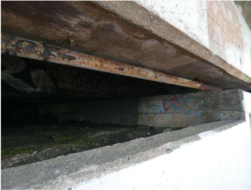
Element: 39 - Services Description: Corrosion on service pipe
