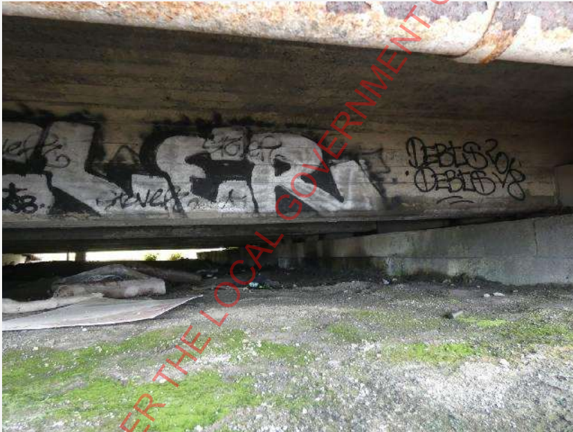
Element: 40 - Appearance Description: Graffiti on beams
